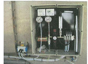
Pneumatic control panel
