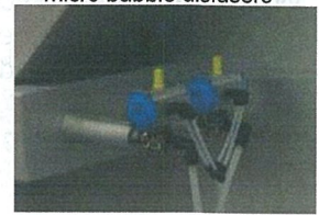
Automatic micro bubble diffuser cleaning system
