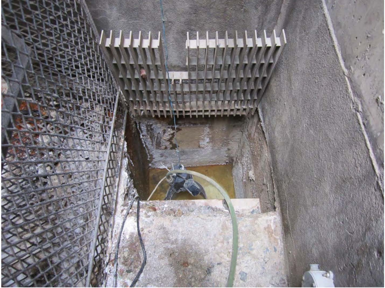
Photo 4 – Sump pump beneath ventilation hatch
