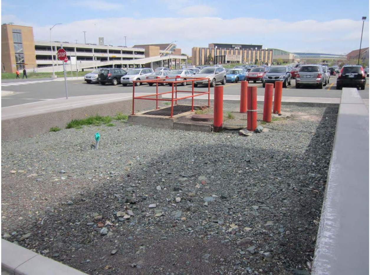
Photo 6 – Ventilation hatch from surface
