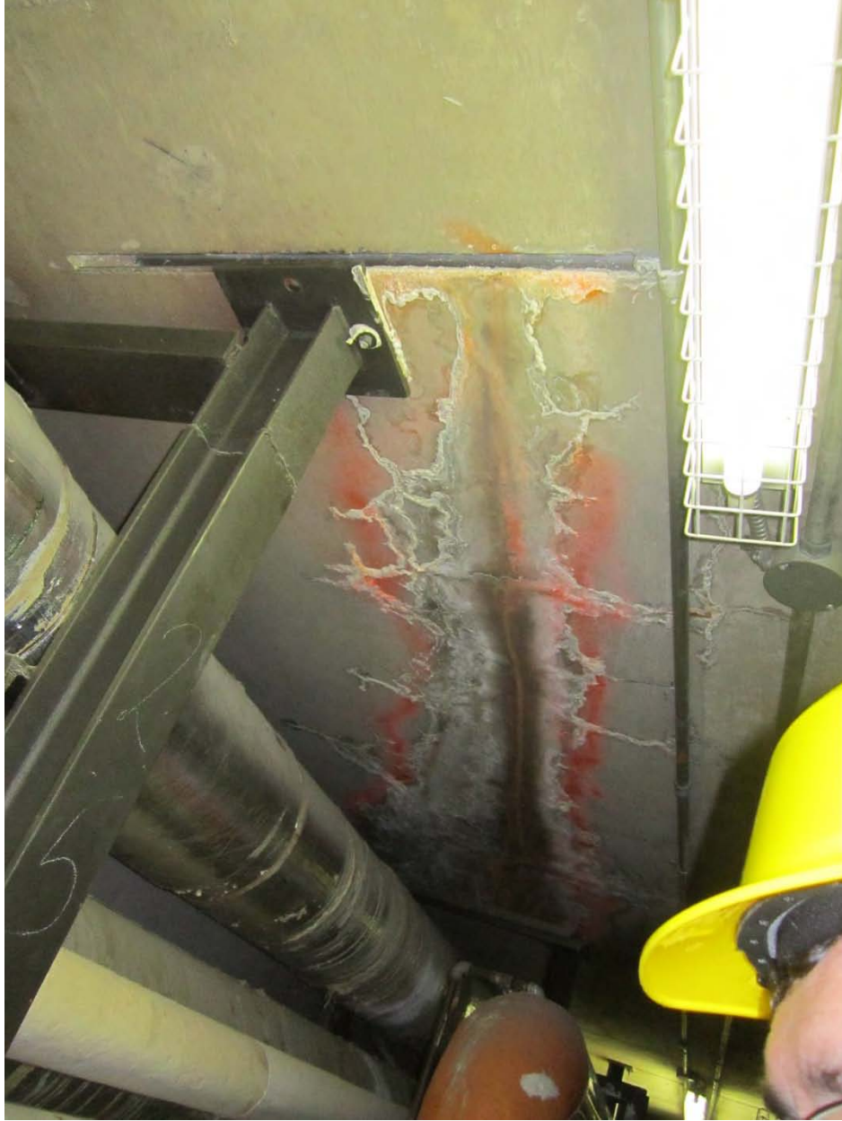
Photo 2 – Tunnel ceiling (observed in only one location)
