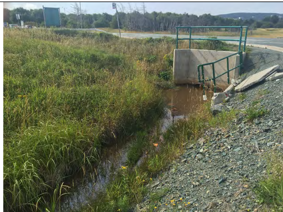
PHOTO 18: Ditch leading to culvert under Clinch Crescent, near southernmost entrance to parking lot. Looking southwest.
