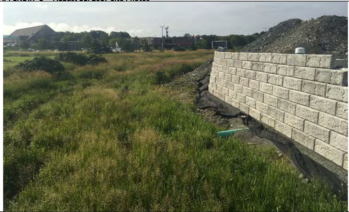
PHOTO 15: Site of initial retaining wall construction, adjacent to Clinch Crescent bridge. Looking south.
