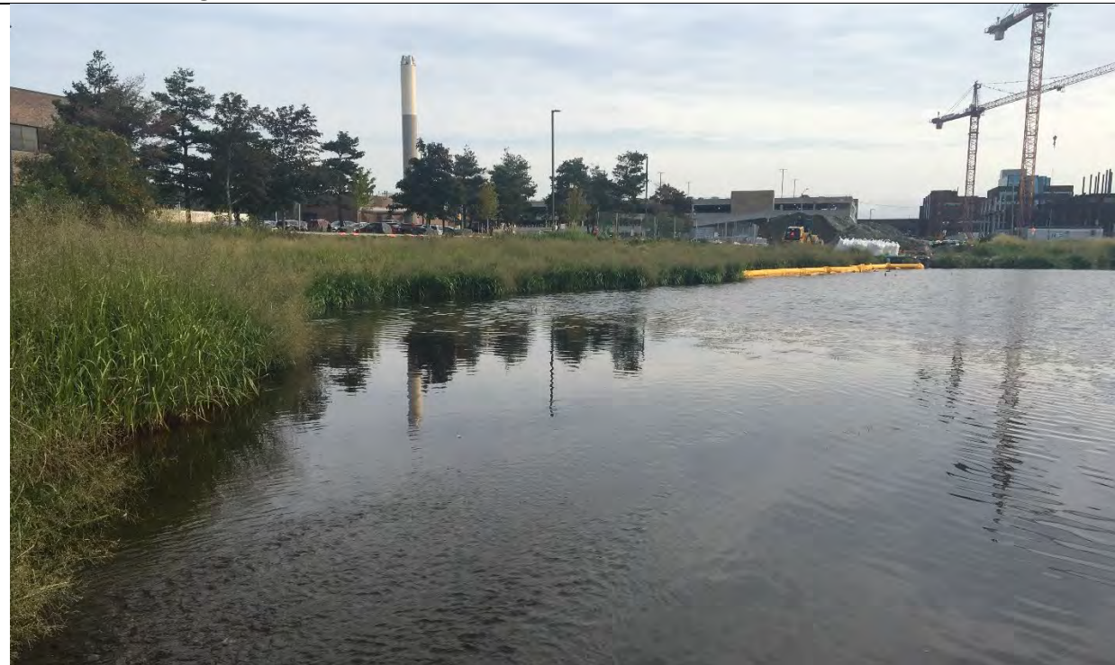
PHOTO 11: Poned area east of the HSC. Sediment control boom visible at site of retaining wall construction. Looking northeast.
