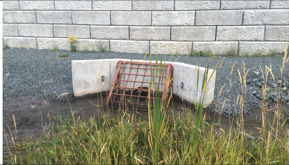
PHOTO 3: Stormwater outflow, presumably from parking areas, discharging into wetland. Looking northwest.
