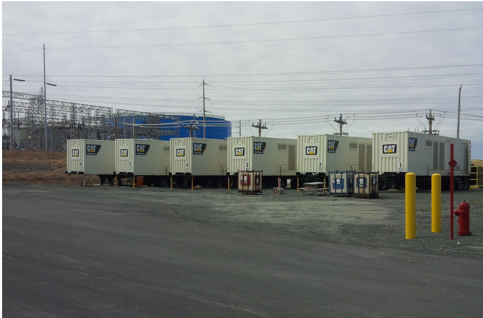
Figure 4: Site Photograph showing the Black Start Diesel Generators
