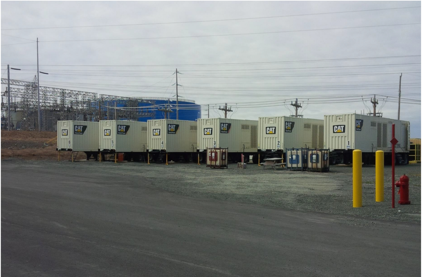
Figure 1.2 Photograph of Mobile Trailers Housing Six – 1.825 MW Diesel Generators at the Holyrood Thermal Generating Station
