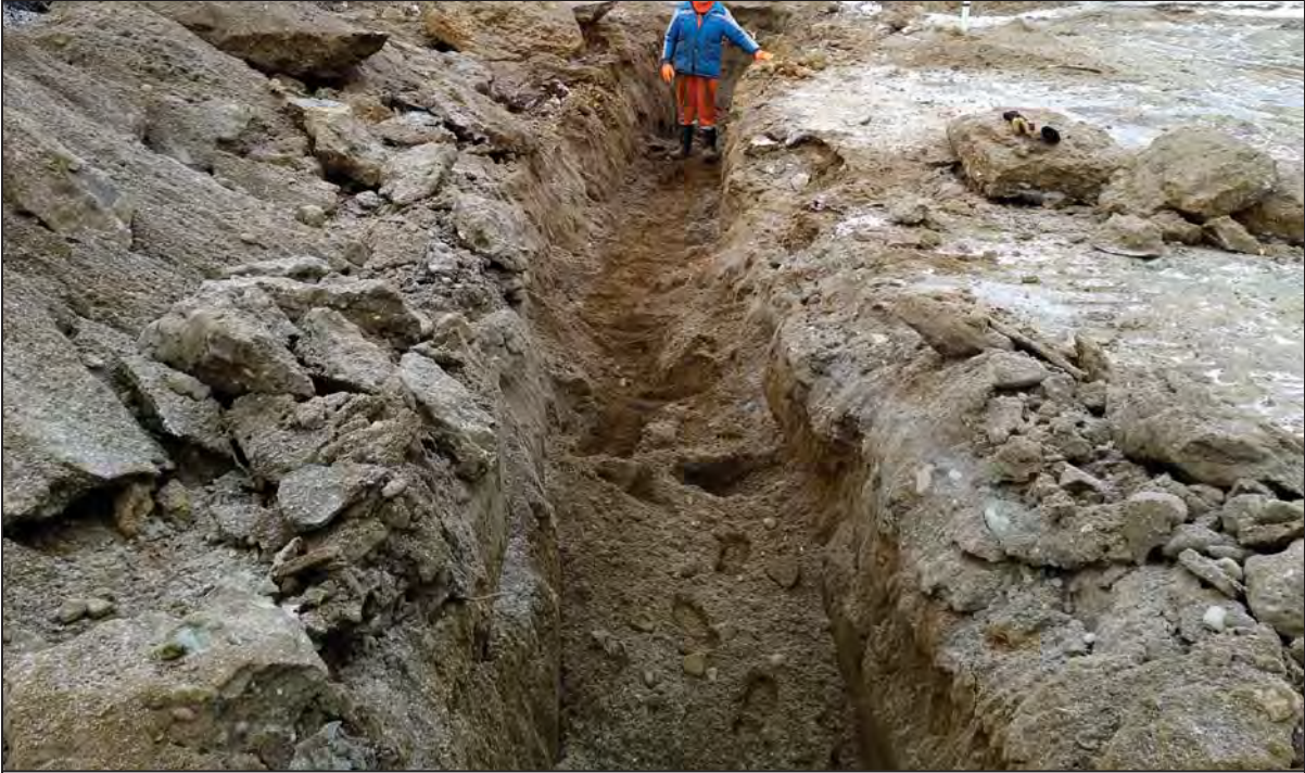
Figure 9 Photograph of staff member standing on the potable water line with the old fuel lines uncovered in the foreground of the slit trench.
