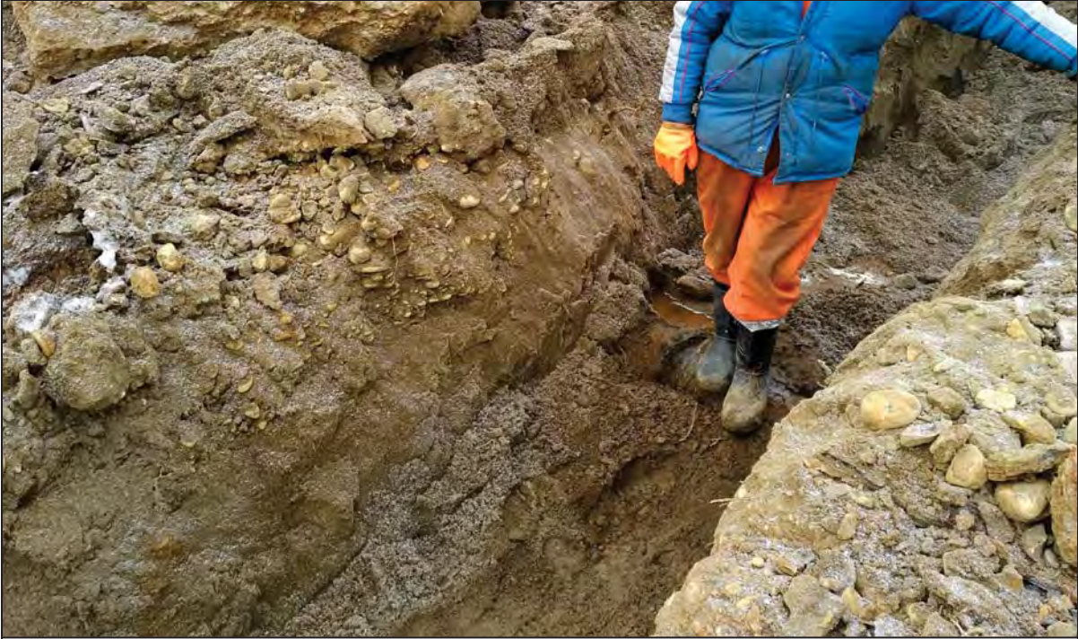
Figure 7 Photograph of staff member standing on the exposed potable water line.
