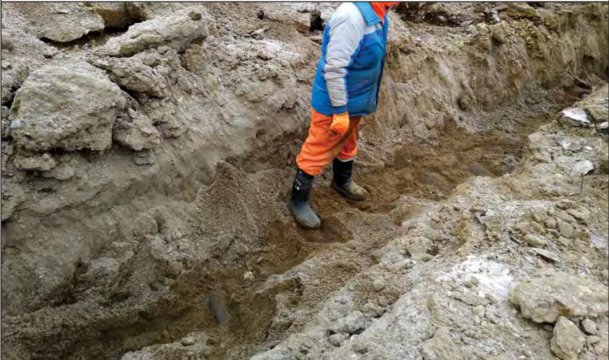
Figure 8 Photograph of staff member standing on two (2) of old fuel lines uncovered in the slit trench with a third line to the staff member's right and two to his left.
