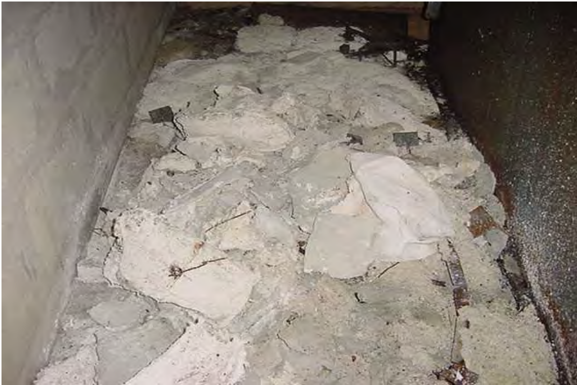
Photo D: View of asbestos containing material in receiver building.
