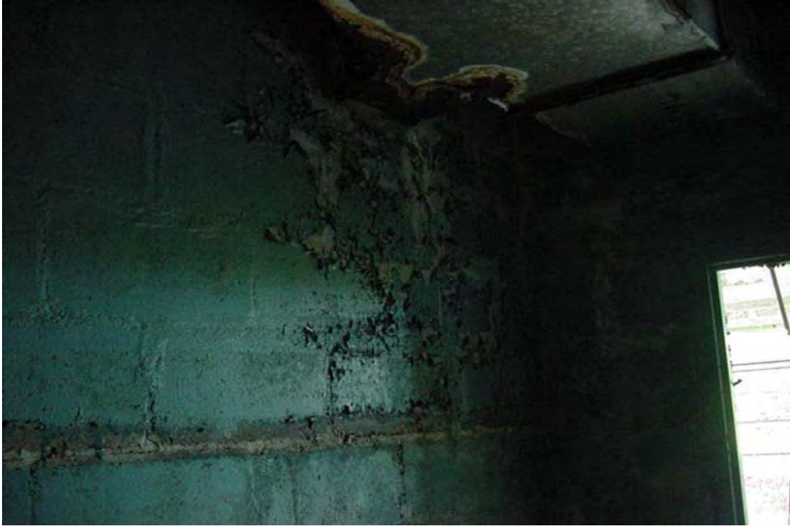
Photo C: View of flaking paint in receiver building.
