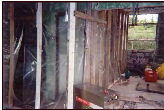
PHOTO 1: VIEW OF ENCLOSURE IN RECEIVER BUILDING.
