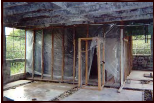
PHOTO 1: VIEW OF ENCLOSURE IN TRANSMITTER BUILDING
