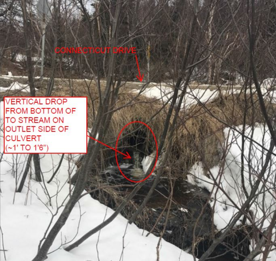
Figure 8: Vertical Separation of Stream at Culvert Location
