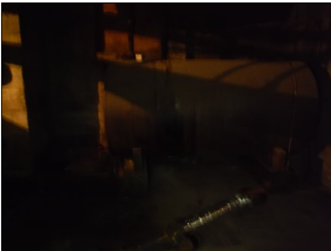
Old, inactive AST (unknown volume) in the basement of the site building
