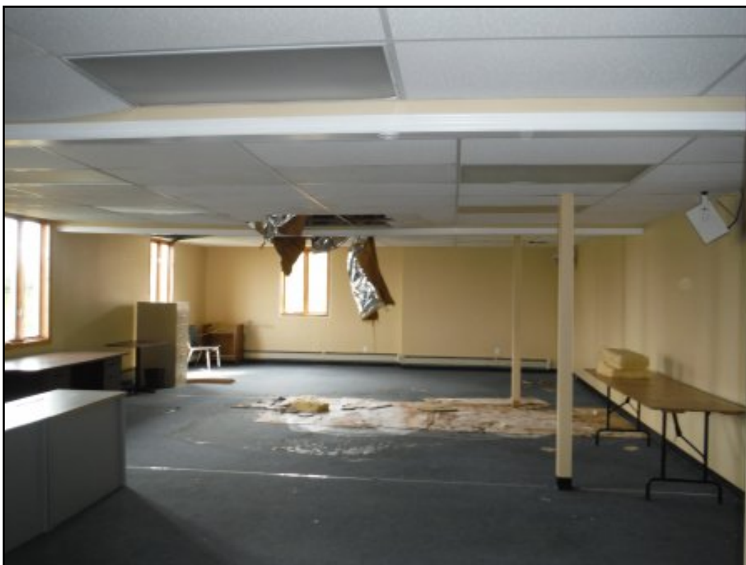
Water damaged materials in the former Academy Canada portion of the site building
