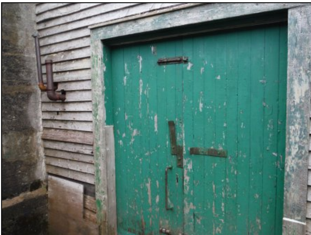
Fill and vent pipes on the north wall of the site building
