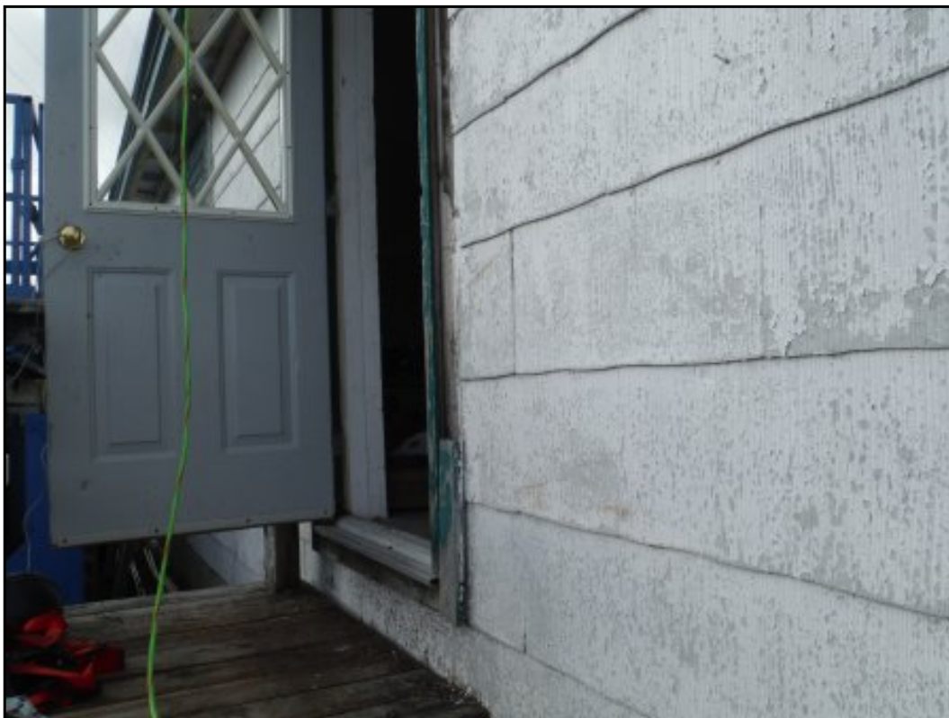
Potential asbestos-containing exterior siding on the southeast side of the site building
