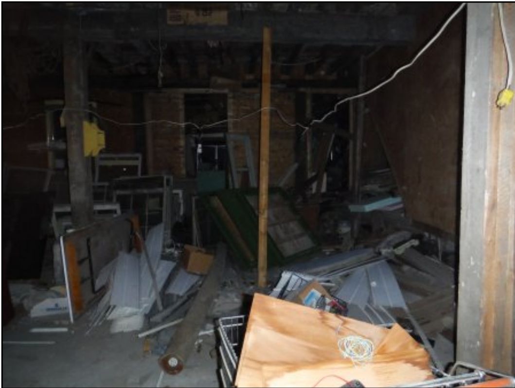
Storage of miscellaneous materials in the basement of the site building
