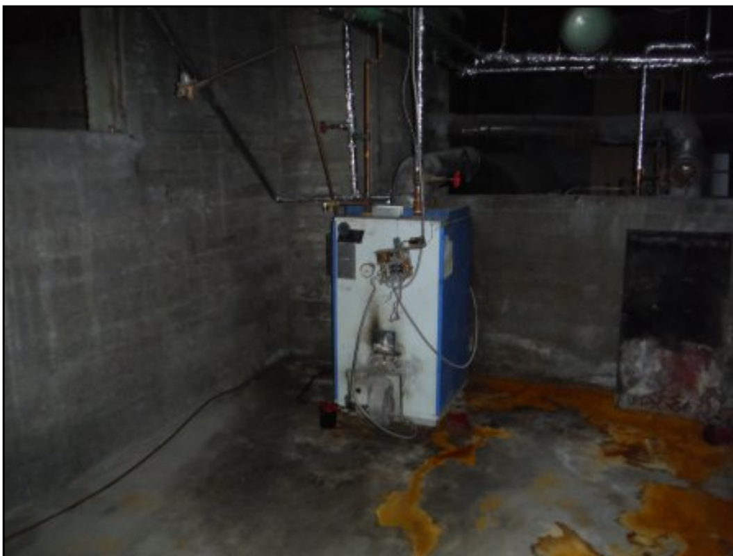
Rust-like staining on the concrete floor of the site building
