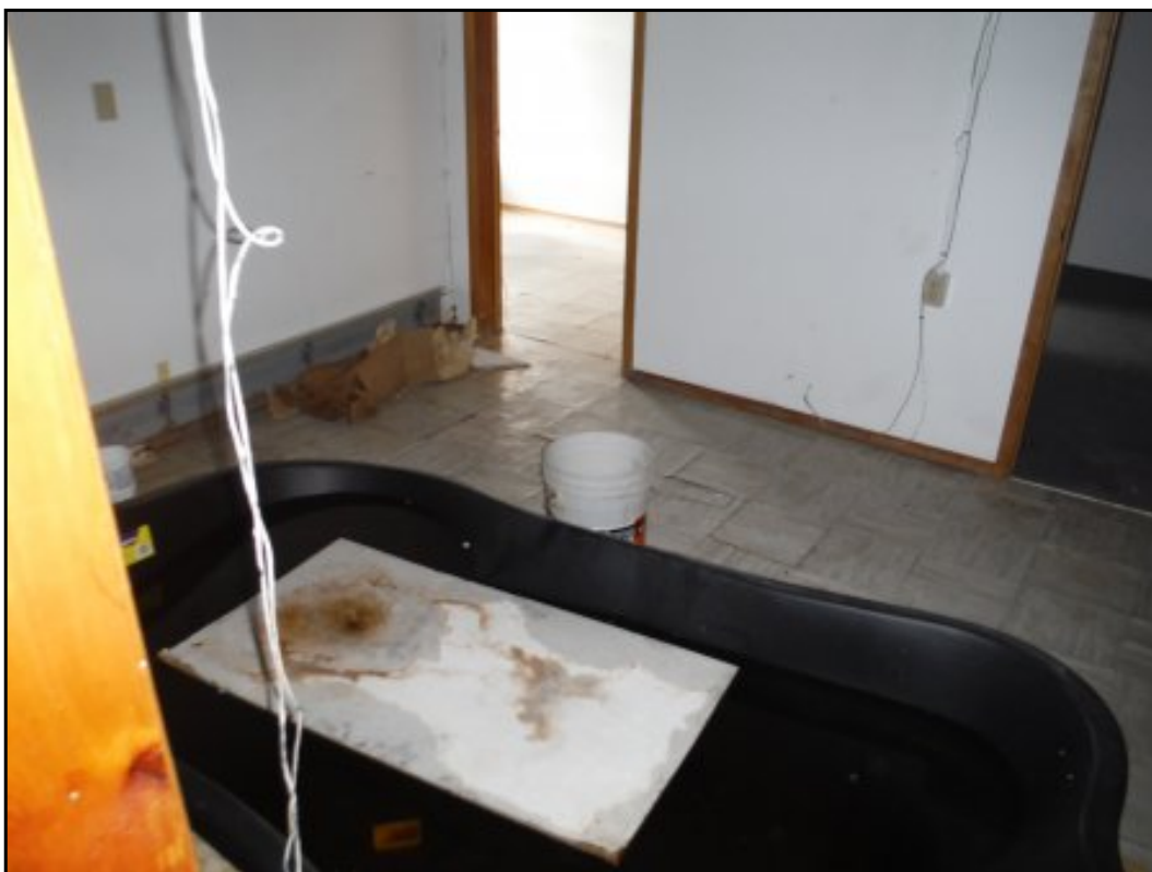
Evidence of water intrusion into the site building
