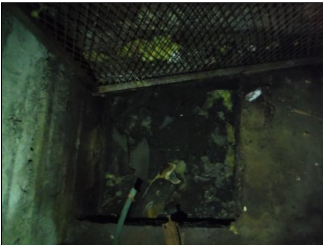
Pit in floor of the basement of the site building, adjacent to the large AST
