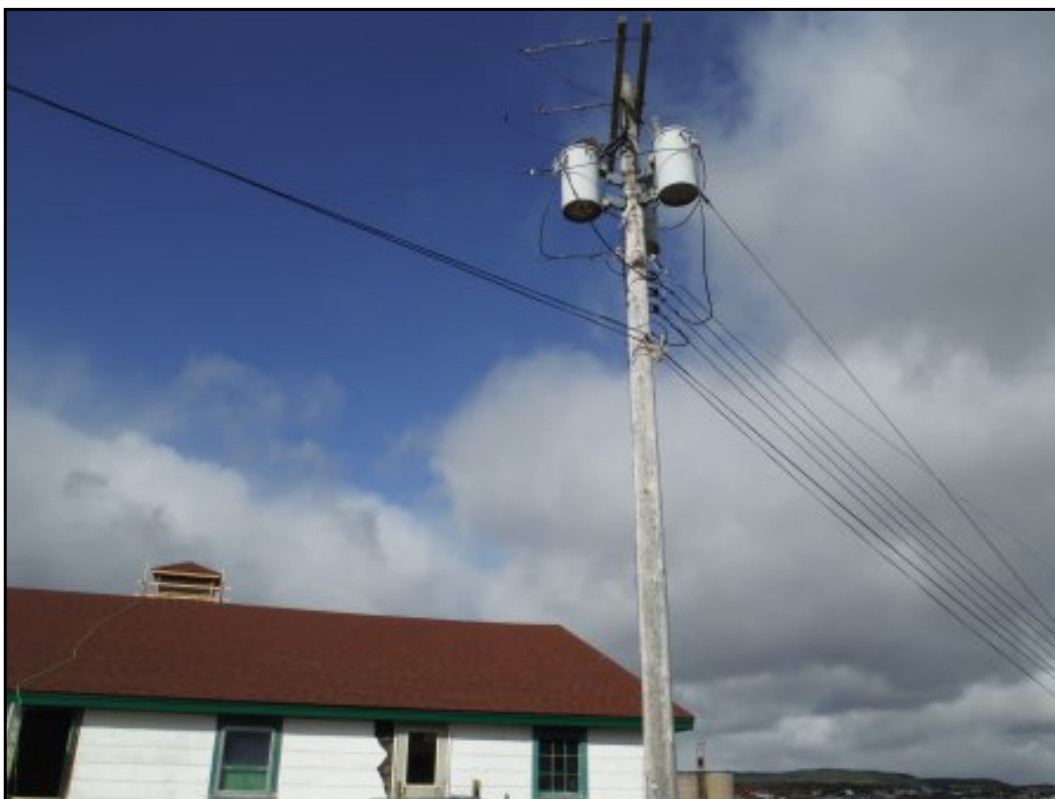
Transformers located on the northeast portion of the Site, looking northwest
