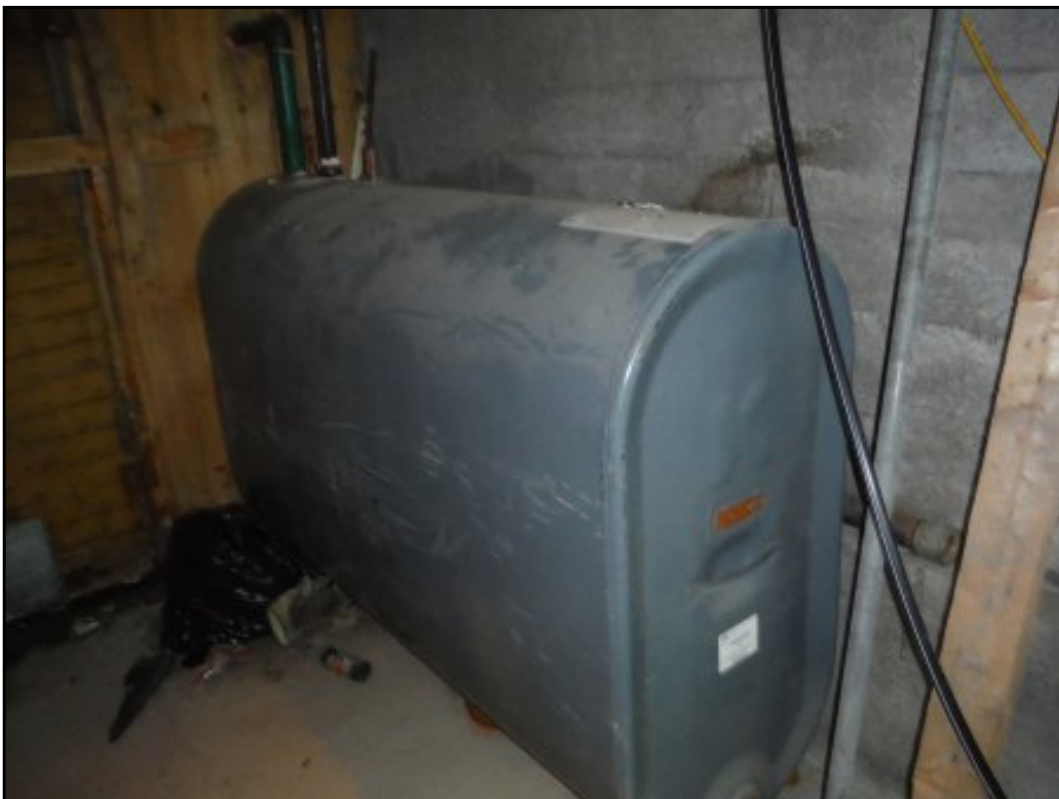
Inactive 1,137 L AST in the basement of the site building
