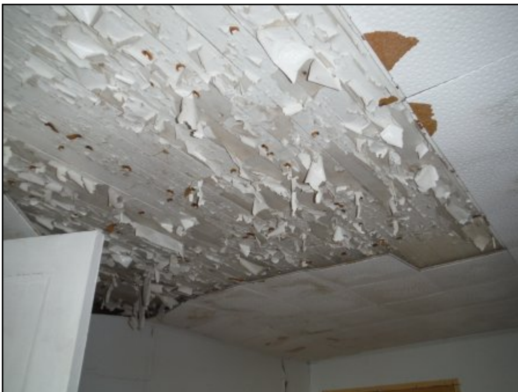
Evidence of water damage and peeling paint in the site building
