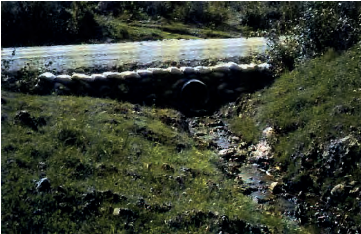
Figure 4.10 Cross drainage culverts and take-off ditches carry water away from the road and into surrounding vegetation.
