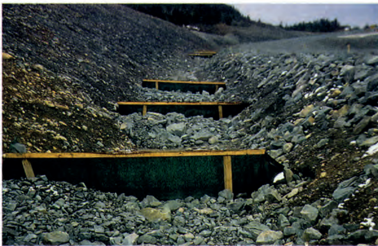
Figure 4.3 Filter fabric dams used in series maximize the effectiveness of the removal of suspended sediment from collected water.
