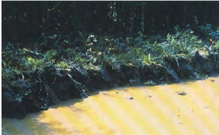
Figure 4.12 Development activities can de-stabilize streambanks, resulting in streambank erosion and considerable sedimentation of watercourses.
