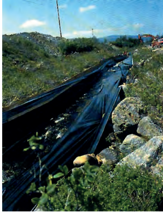
Figure 4.35 Temporary diversion channels should be lined with plastic that is weighted down with stone.
