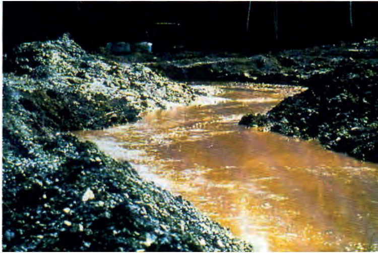
Figure 4.1 Development activities can lead to the erosion of soils into nearby watercourses.
