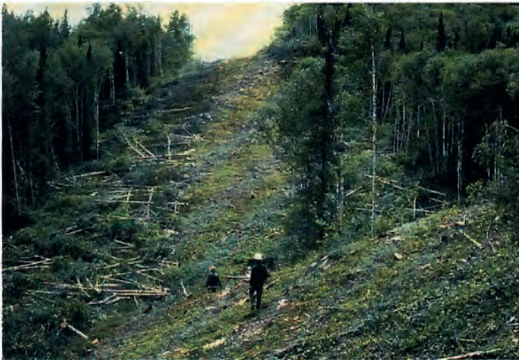
Figure 4.31 Right-of-way clearing and grubbing is commonly associated with many construction developments, including roads, pipelines and transmission lines.
