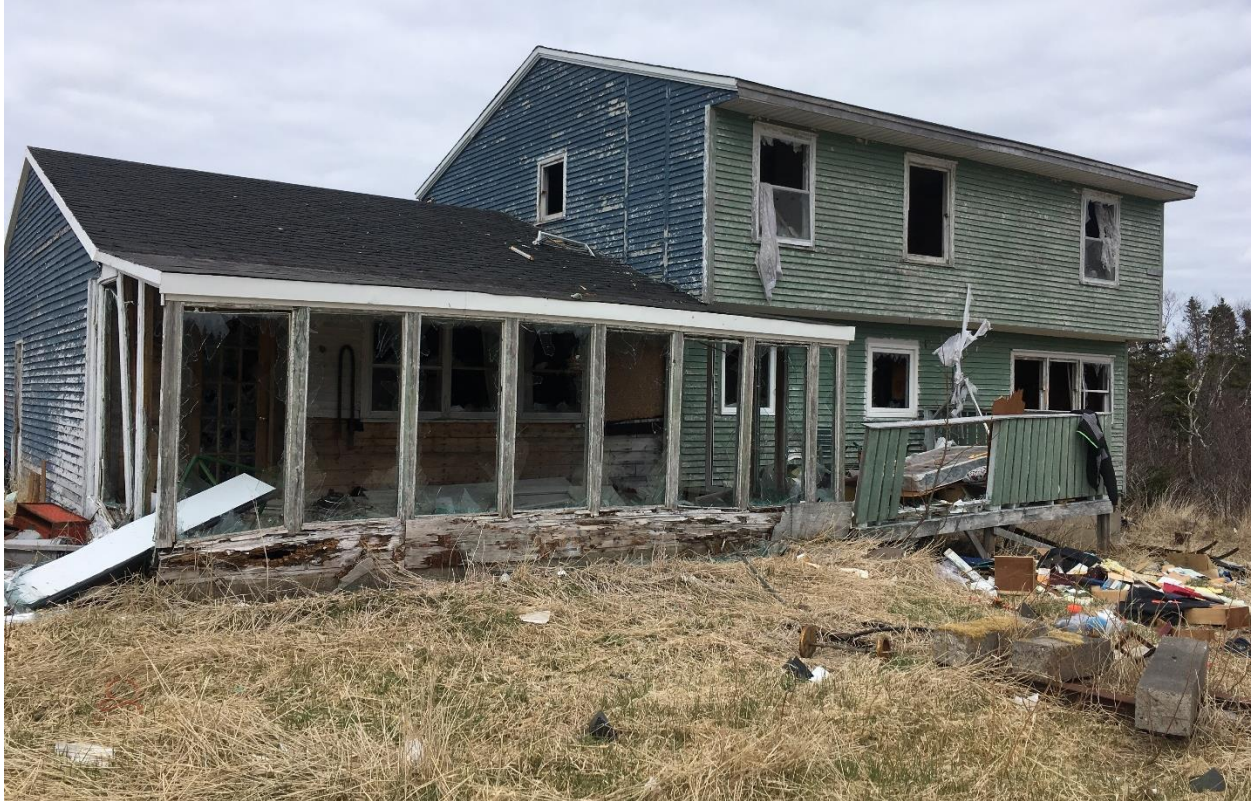
Figure 12: Abandoned Building on Crown Land Grant
