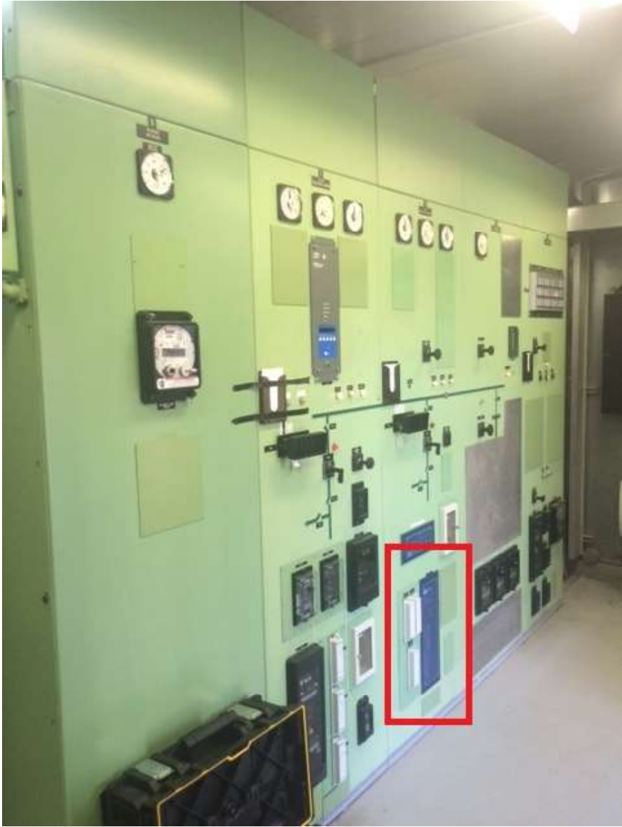
Figure 10 Location of Relay Switch inside Terminal Station Building
