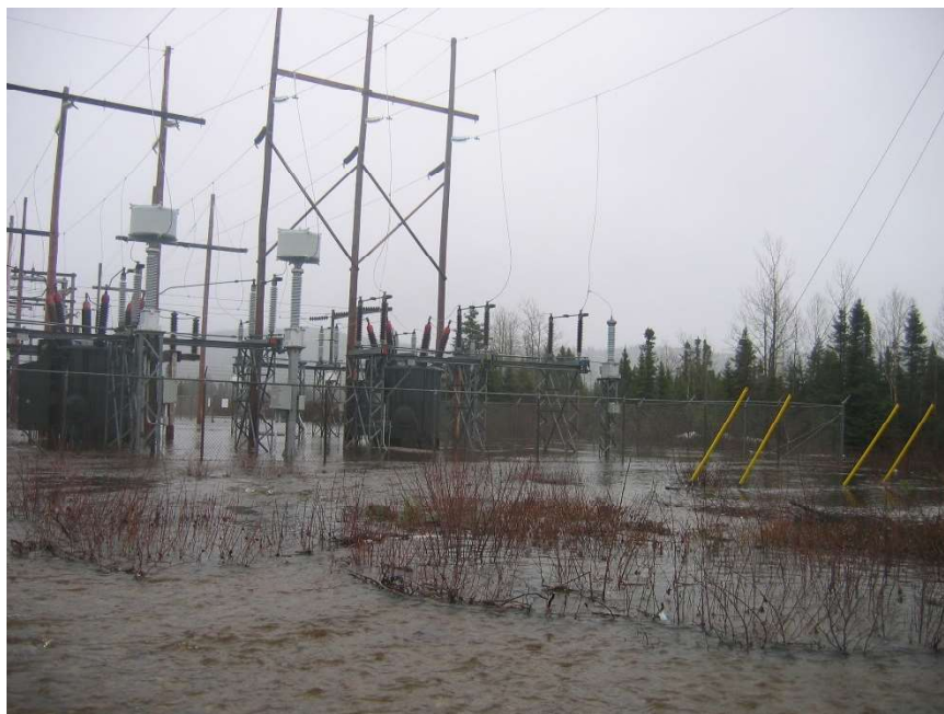
Figure 7 Flooding at Terminal Station (April 18, 2006) – Photo 4
