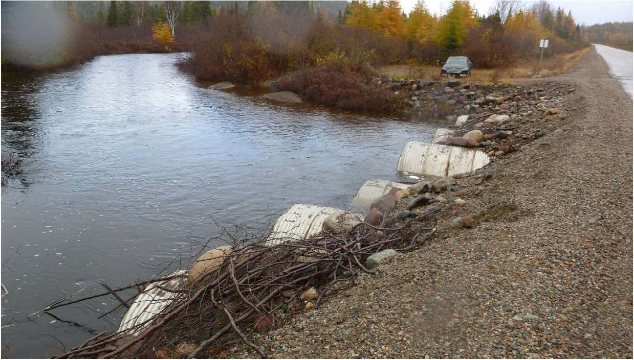
Photo 3: Woody debris at upstream of culverts at route 392.
