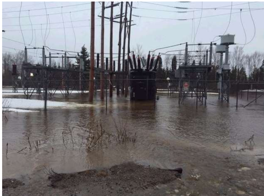
Figure 9 Flooding at Terminal Station (April 29, 2015) – Photo 2
