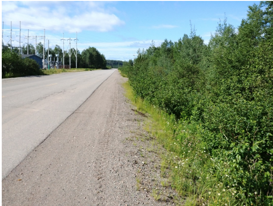
Figure 14: Option 2 Site Visit Observation 1 – Ditch Heavily Overgrown
