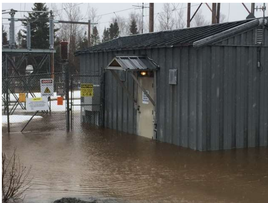
Figure 8 Flooding at Terminal Station (April 29, 2015) – Photo 1
