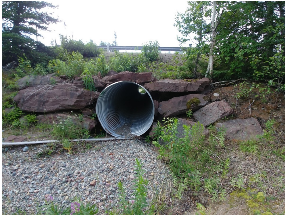
Figure 20: Option 2 Site Visit Observation 2f - 1600mm Cross Culvert on Route 390
