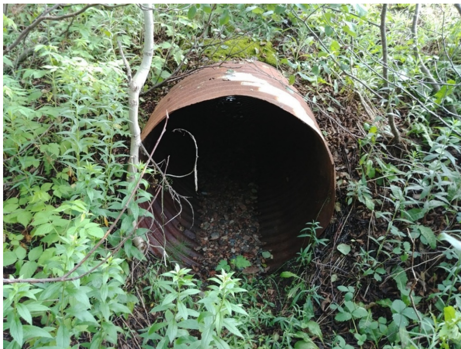
Figure 18: Option 2 Site Visit Observation 2d – 900mm Culvert at Highway Sign Embankment
