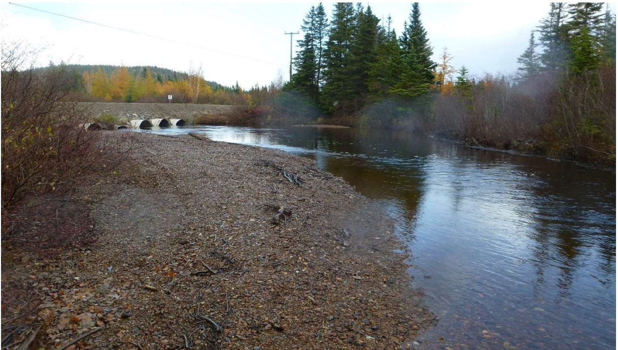
Photo 6: Woody debris and sediment on overbank downstream of culverts at Route 392.
