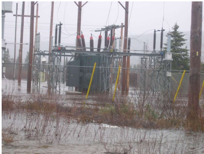
Figure 5 Flooding at Terminal Station (April 18, 2006) – Photo 2
