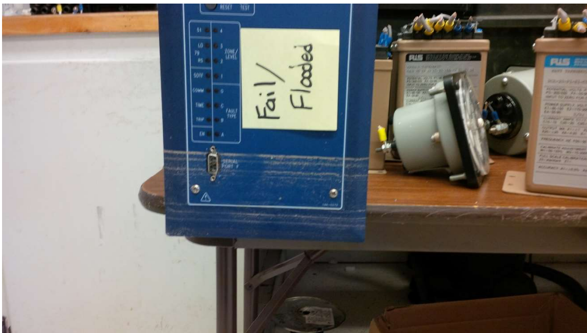
Figure 12 Watermarks on Relay Switch Removed after 2015 Flood
