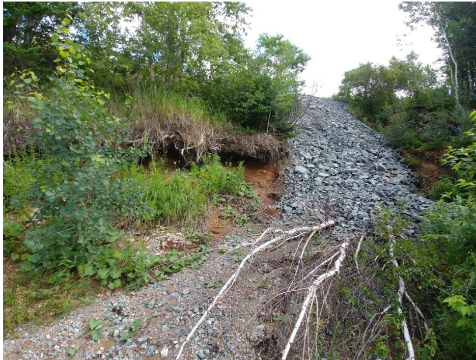
Figure 24: Option 2 Site Visit Observation 6 - Erosion Between Route 390 and Indian River
