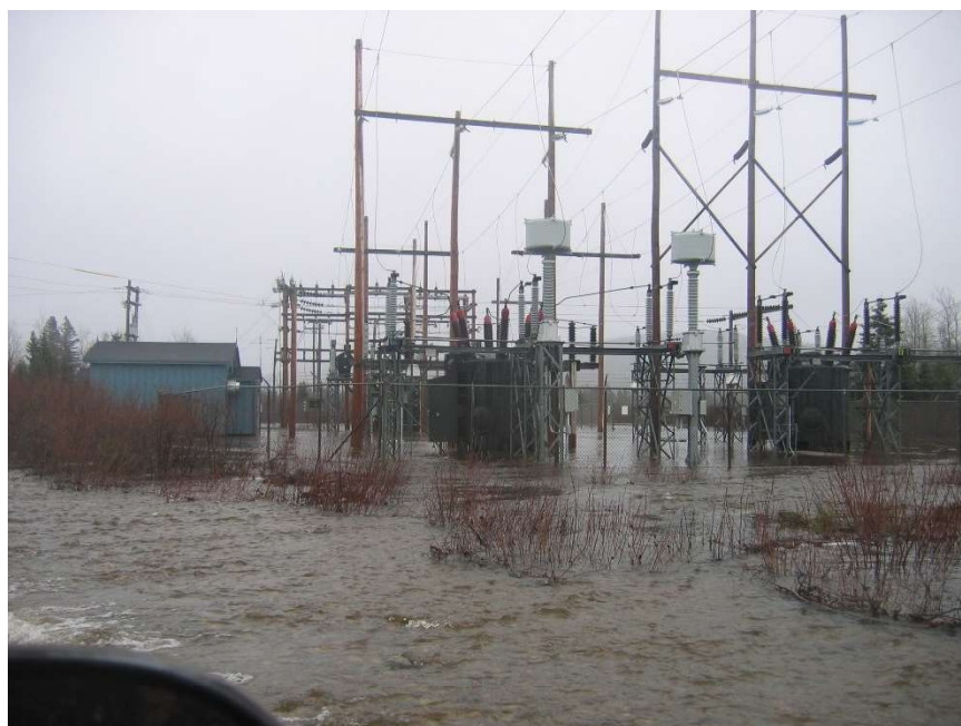
Figure 6 Flooding at Terminal Station (April 18, 2006) – Photo 3
