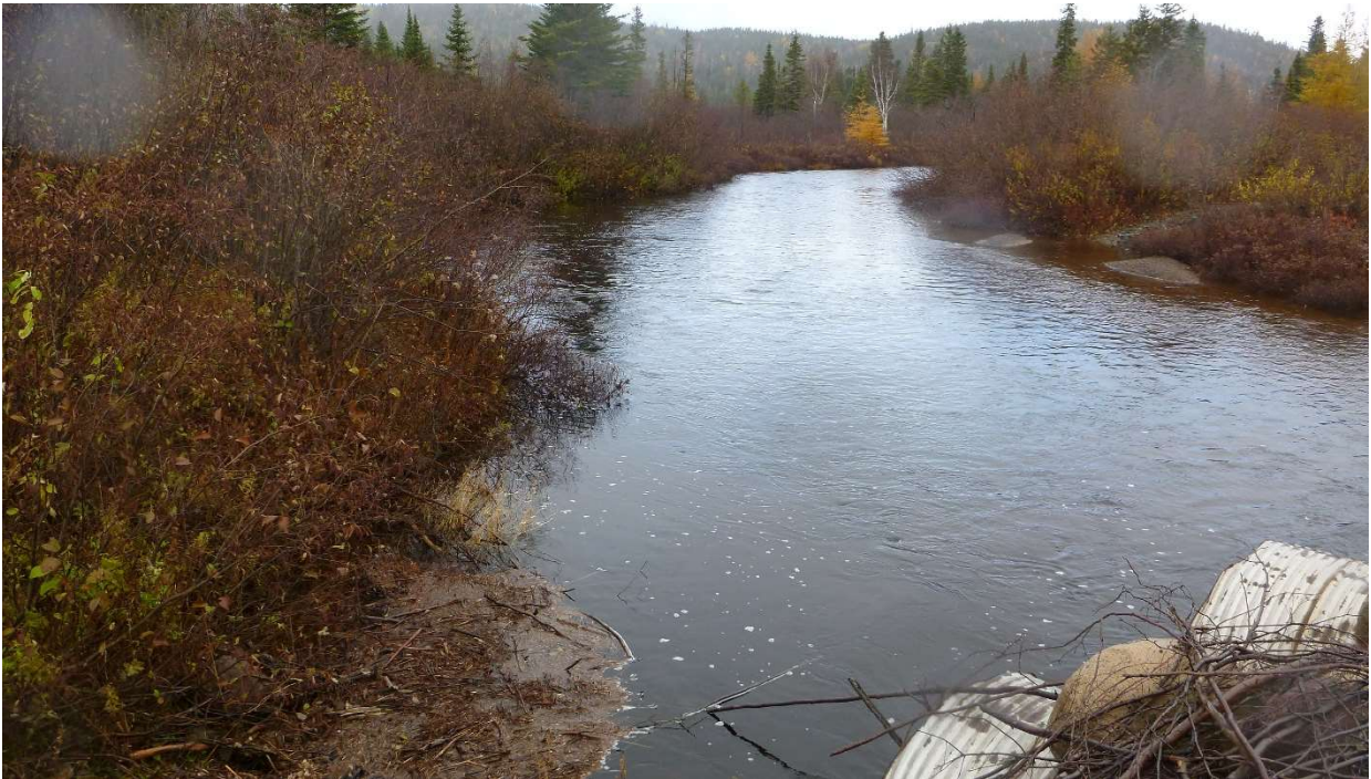
Photo 4: Heavy brush on overbanks upstream of Route 392 culverts.
