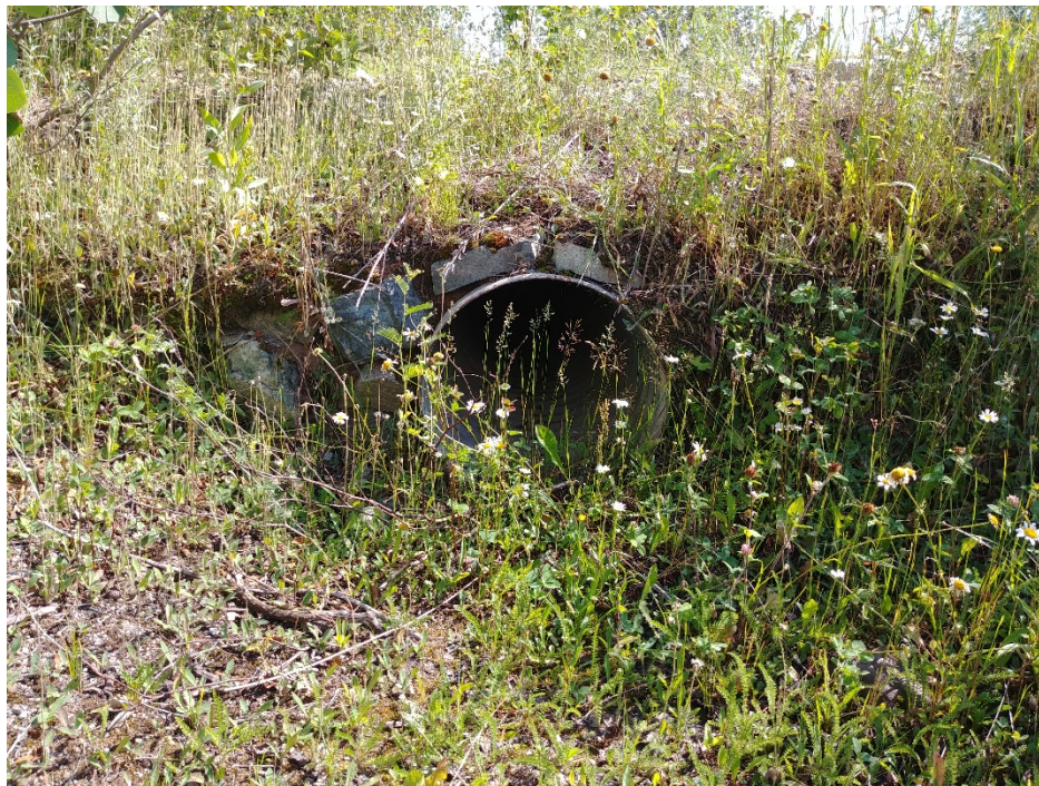
Figure 16: Option 2 Site Visit Observation 2b – 450mm Accessway Culvert Approximately 50m Southwest of Little Bay Road
