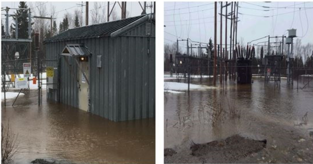
Figure 2-1: Flood Conditions at Springdale Terminal Station
