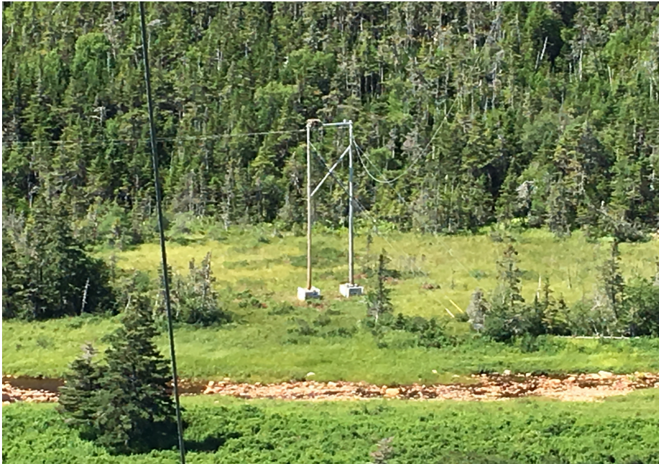
Figure 6-1: Photo of Osprey Nest on Pole 51, west of Bay de L’Eau River
