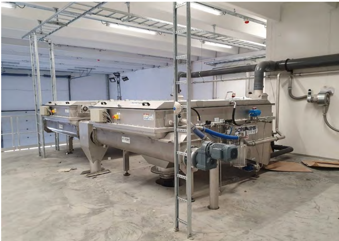
Figure 17: Purification of the Drain Water- Sludge Dewatering Machines
