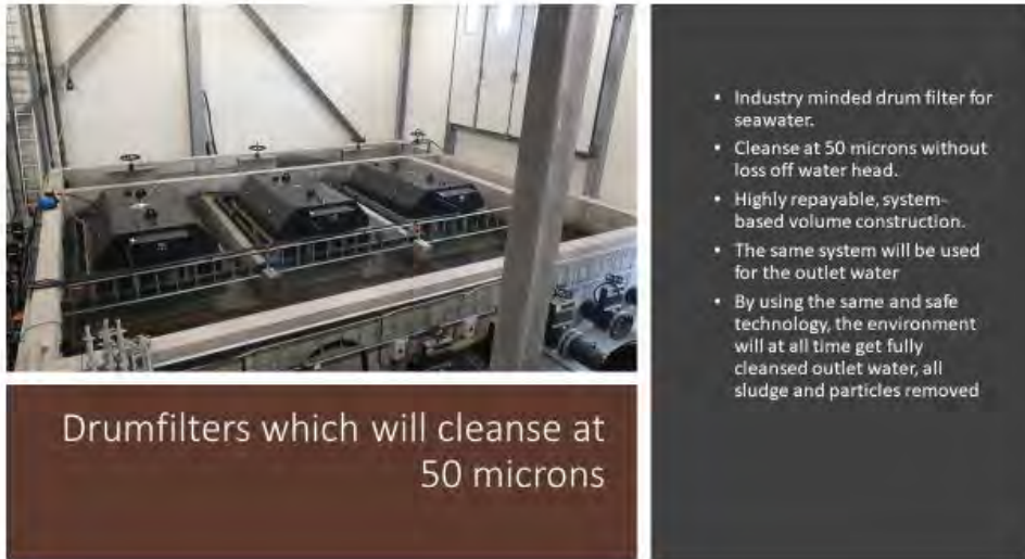
Figure 15: Drum Filters for Filtering Effluent Sea Water at 50 - micron.
