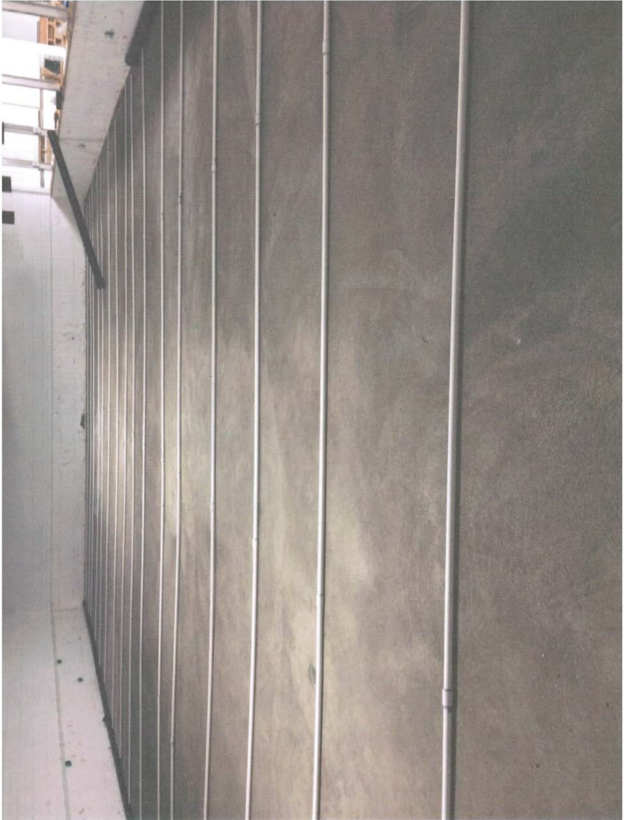
PIPING FOR OXYGEN
