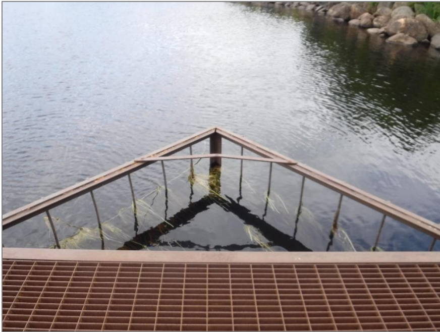
Figure B-6. Trash rack at upstream end of fish ladder (07/14/2016)
