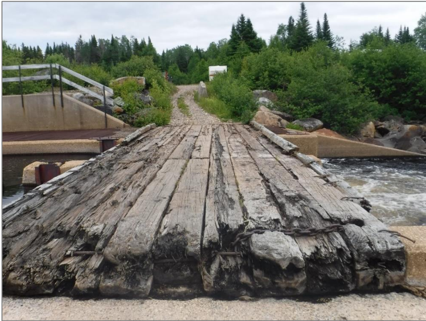
Figure B-4. Decking above fish ladder and spillway, adjacent to access road (07/14/2016)
