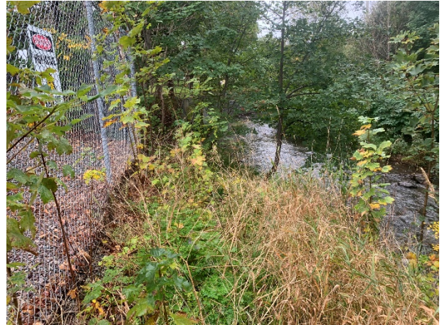
Photo 4: Berm 2 - Rennie's River looking west and fence line of electrical substation adjacent to Kings Bridge road.
