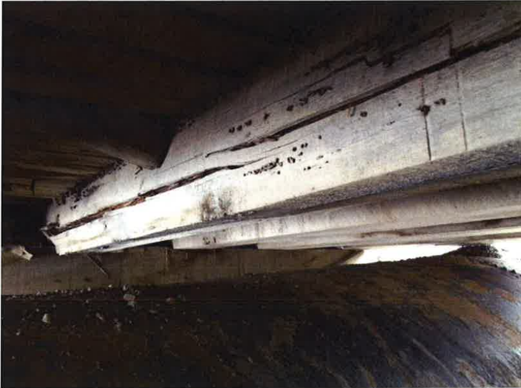
Longitudinal Damage to Beam 4
