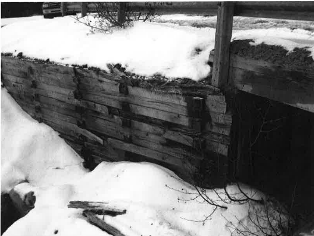
South East Wing Wall - Delamination
