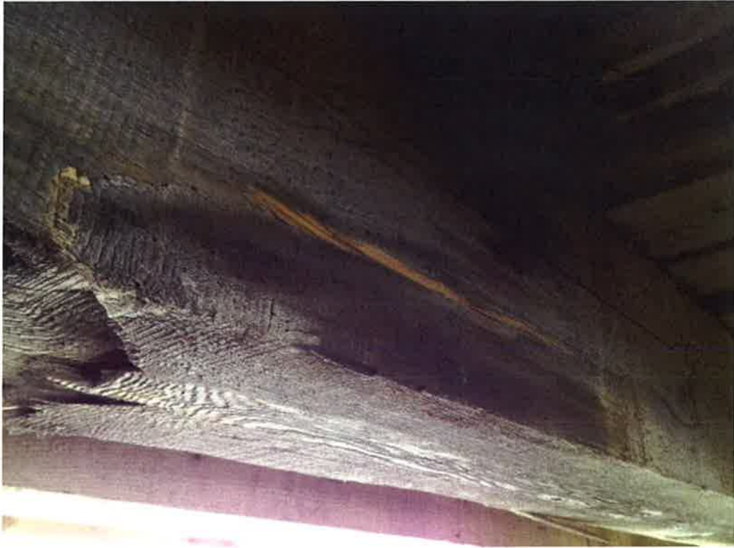
Longitudinal Damage to Beam 6 - Near Mid-Span
