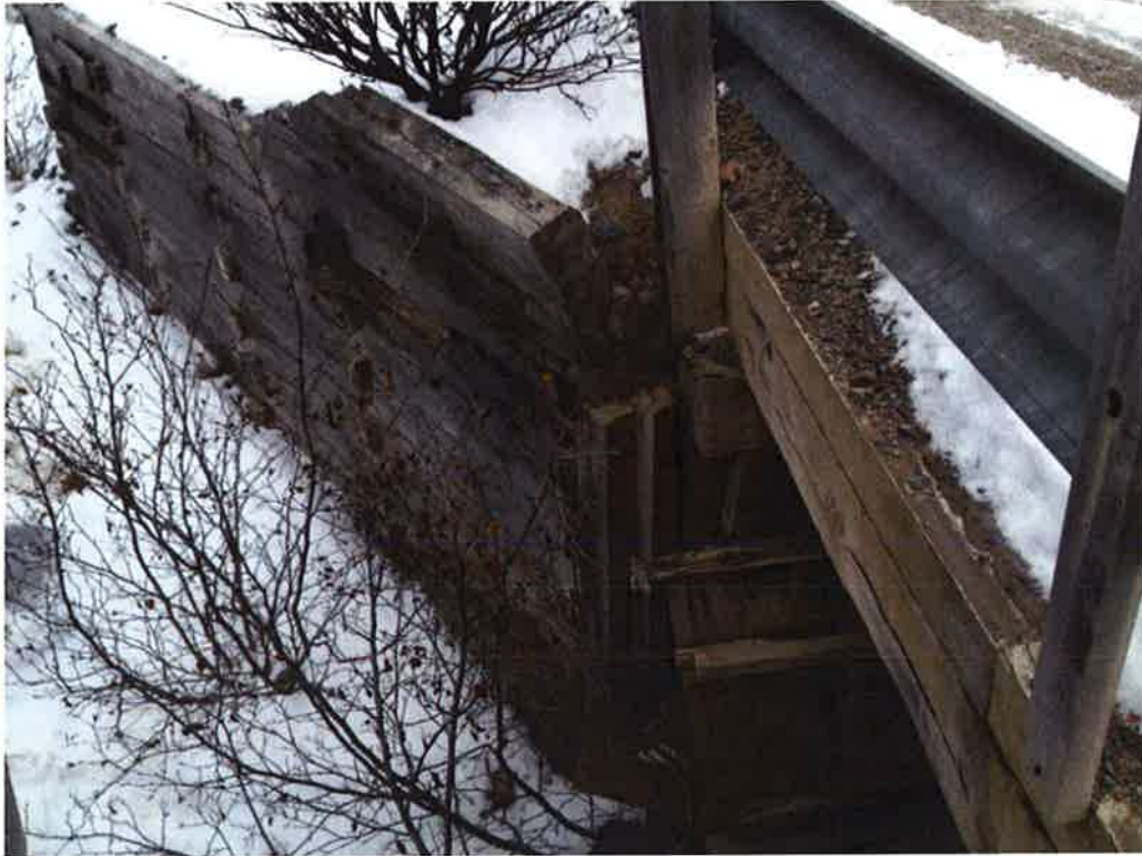
North West Wing Wall - Some Deformation at Top
