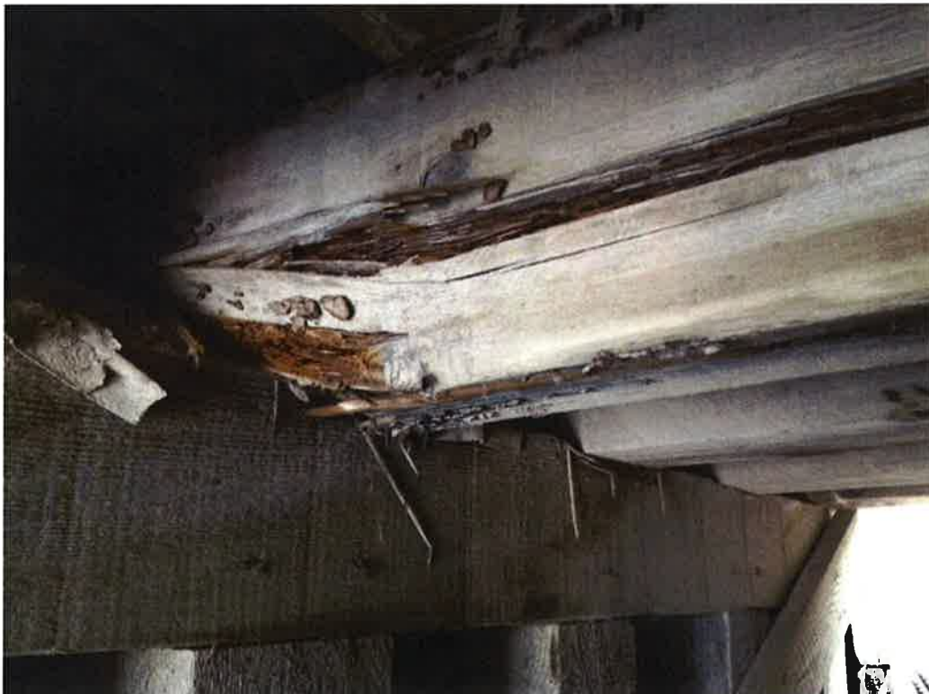
Bearing and Shear Damage to Beam 4 - South End
