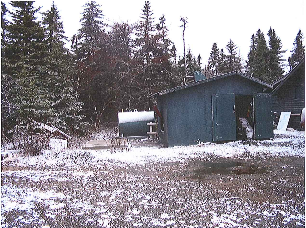
Photo#2: Looking southwest at generator shed, with shop at right. Note concrete pad at left-location of new diesel AST.
