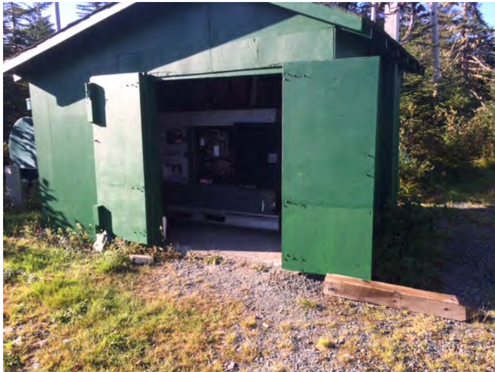
Photo 4 – View, looking south towards the generator shed during the September 2018 Site inspection after the generator shed after rot was repaired on the lower right door.
