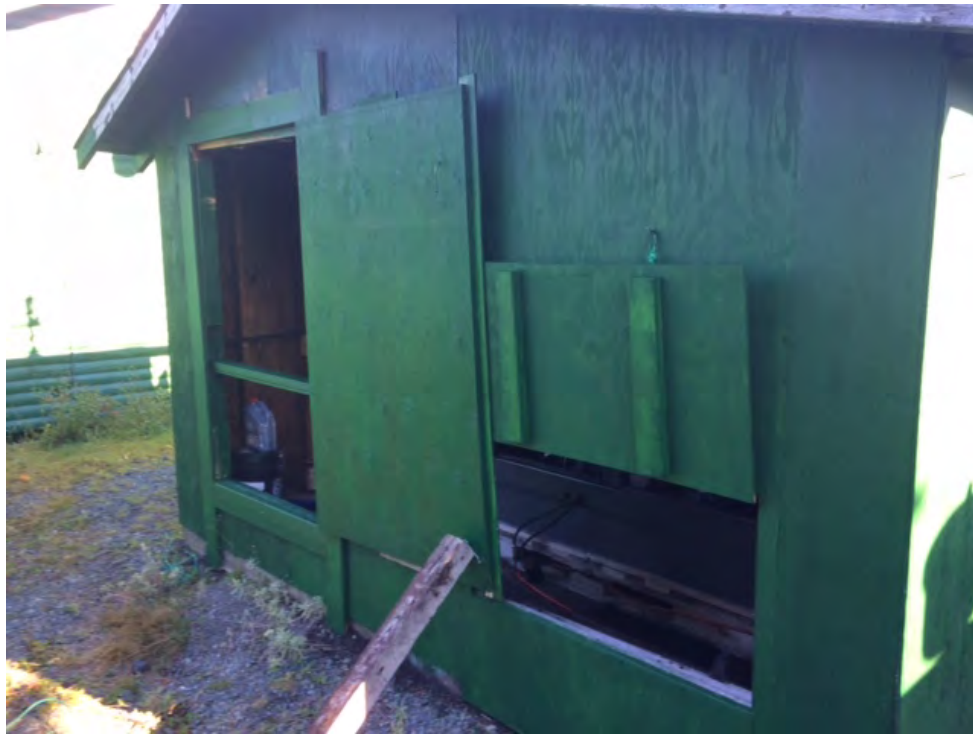
Photo 3 – View, looking northwest towards the generator shed and workshop during the September 2018 Site inspection after the generator shed repairs and painting.
