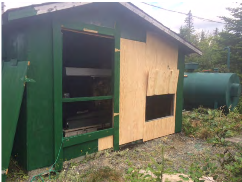
Photo 2 – View, looking east, that shows replacement of the petroleum impacted shed wall during the August 2018 Site inspection.
