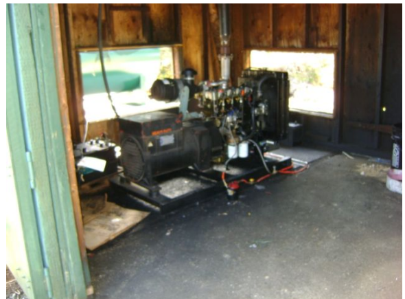
Photo 6: View of the generator owned by the park.
