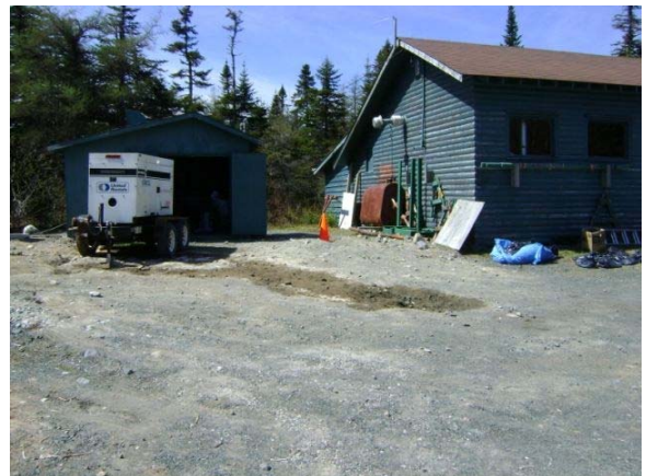
Photo 14: View of the location of the United Rentals diesel generator and the area of surface staining.
