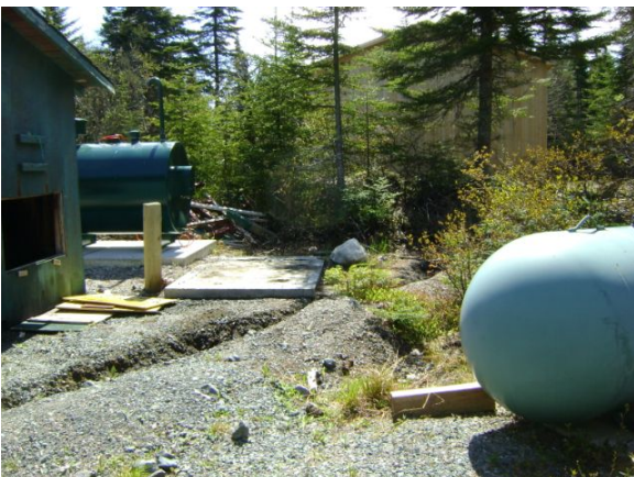
Photo 7: View of the concrete pad for the existing diesel AST and the concrete pad for the historic AST.
