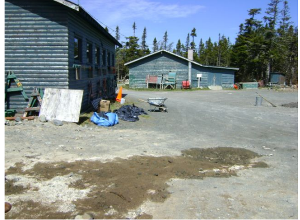
Photo 12: View of the diesel generator spill area and garbage bags containing impacted soil.
