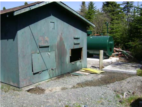
Photo 15: View of the area of surface staining on the south side of the generator shed.
