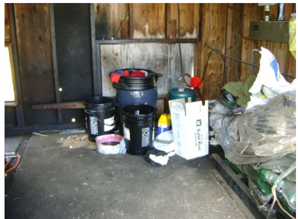
Photo 16: View of oil storage containers and staining on the concrete floor of the generator shed.
