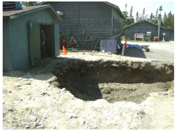
Photo 18: View of the remedial excavation on the north side of the generator shed.
