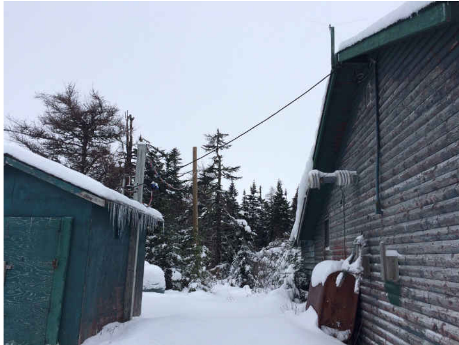
Photo 4: Low hanging power lines between generator shed and workshop.
