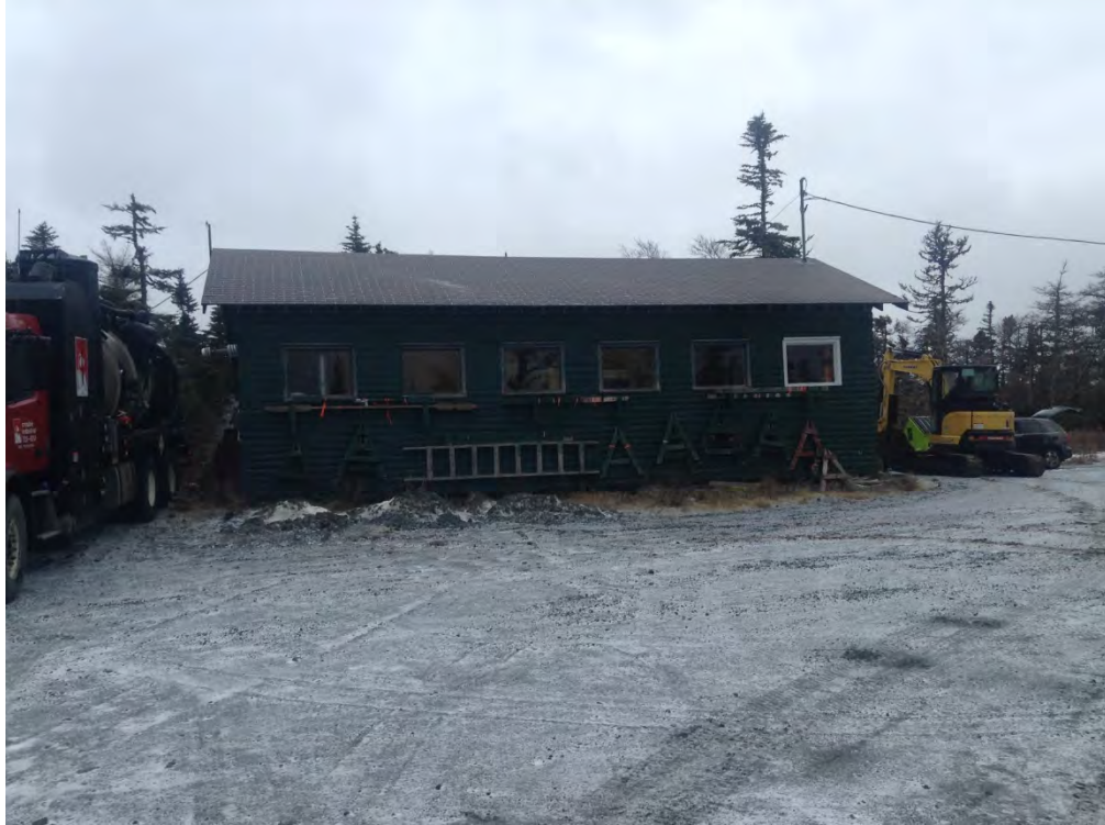
Photo 1 – View, looking southwest towards the workshop, note the Hydrovac truck and excavator (completing TP1) in the background.
