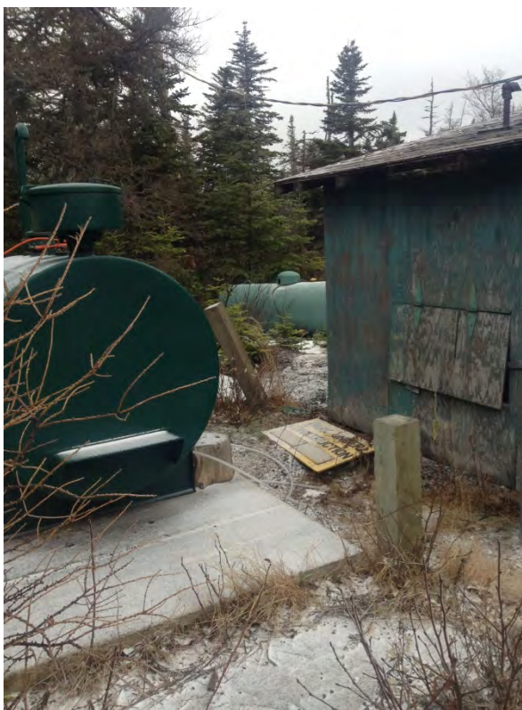
Photo 5 – View, looking southwest at side of generator shed, note the diesel fuel AST and the propane AST.
