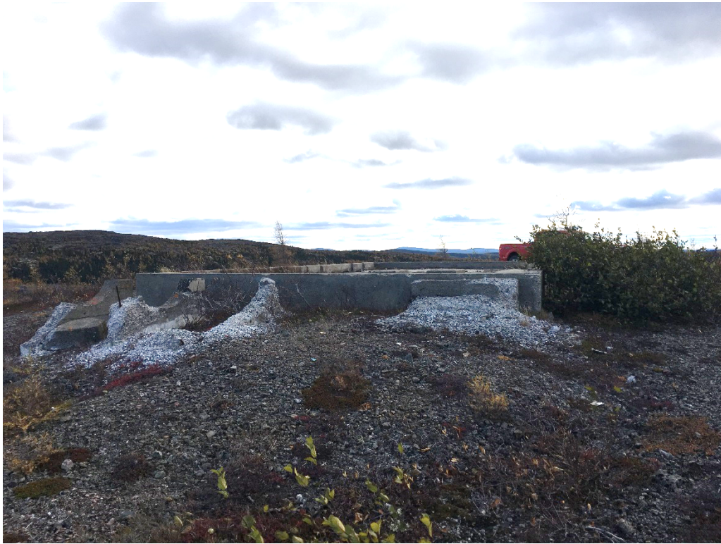
Photo 9 – Former USAF Dump Area and Ammunition Storage Area: foundation of former ammunition storage building. Looking east.
