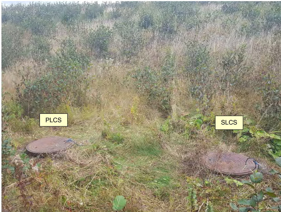
Photo 6 - View, looking east, showing the PLCS and SLCS chambers during the October 2017 monitoring event.
