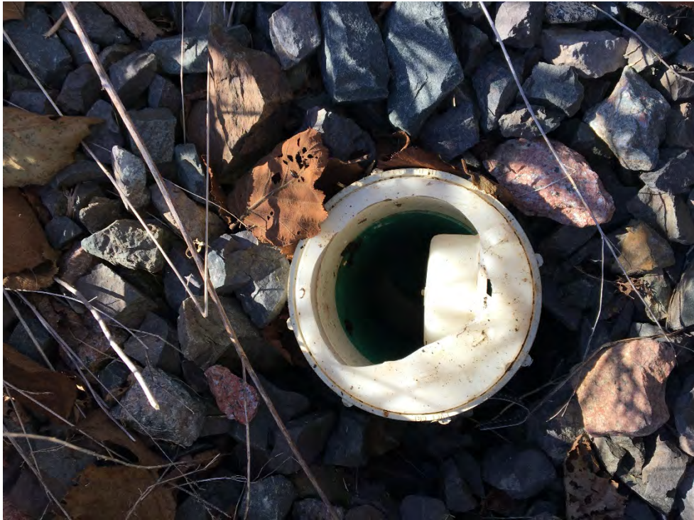
Photo 11 - View of groundwater drainage system clean out CO2. Note the 4" drain cap is damaged.
