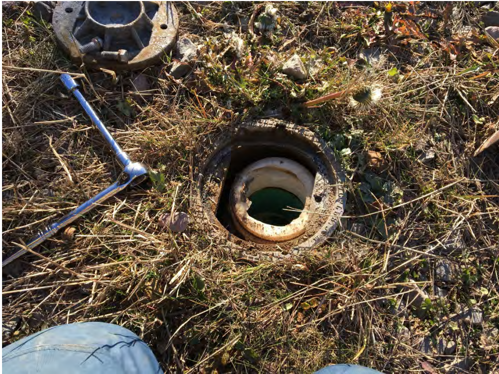
Photo 12 - View of groundwater drainage system clean out CO4. Note the 4" drain cap is damaged.
