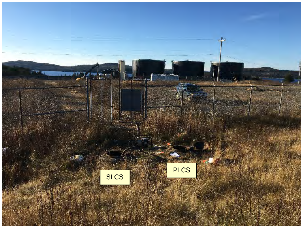
Photo 14 - View, looking west, while pumping leachate from the PLCS and SLCS chambers in November 2017.
