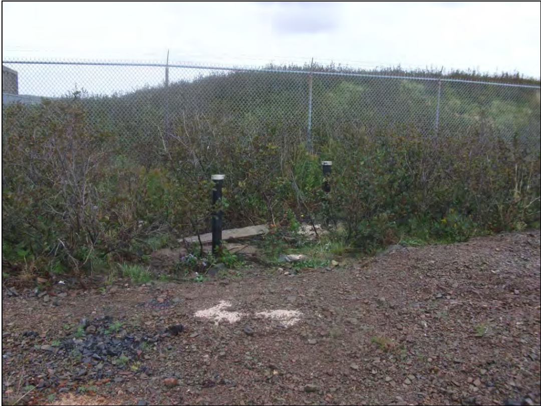
Photo 2: View, looking northeast, of the newly installed groundwater monitor wells (MW10-1 and MW10-1A).
