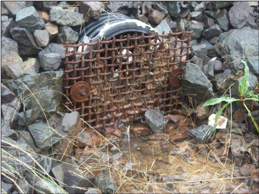
Photo 10: View, looking northeast, showing groundwater discharge from the groundwater drainage system beyond the service road.
