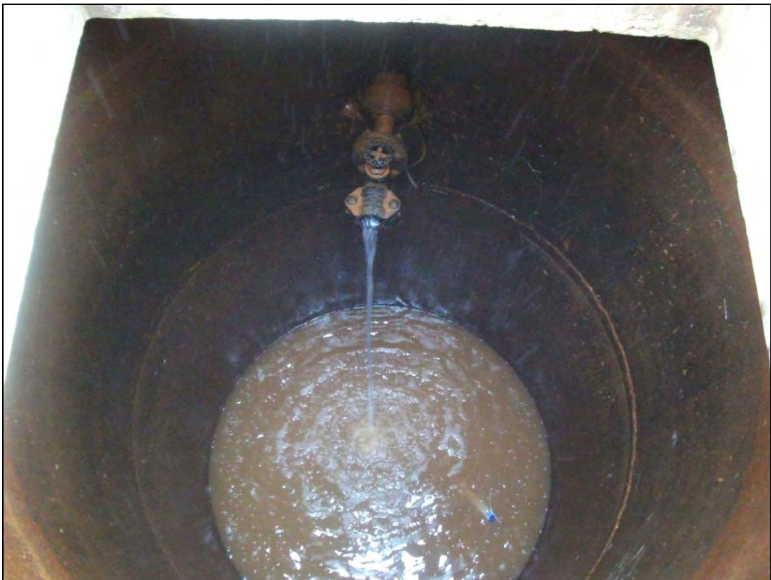
Photo 4: View of PLCS valve chamber with discharge hose disconnected.
