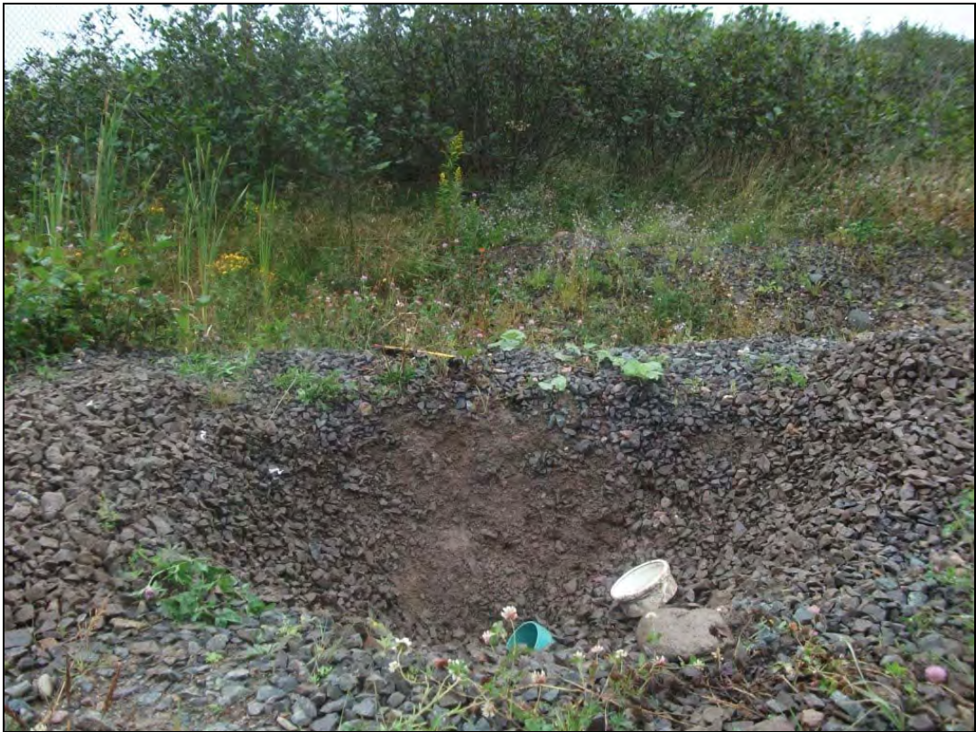
Photo 8: View, looking southeast, showing Clean-out 2 prior to modifications (typical).
