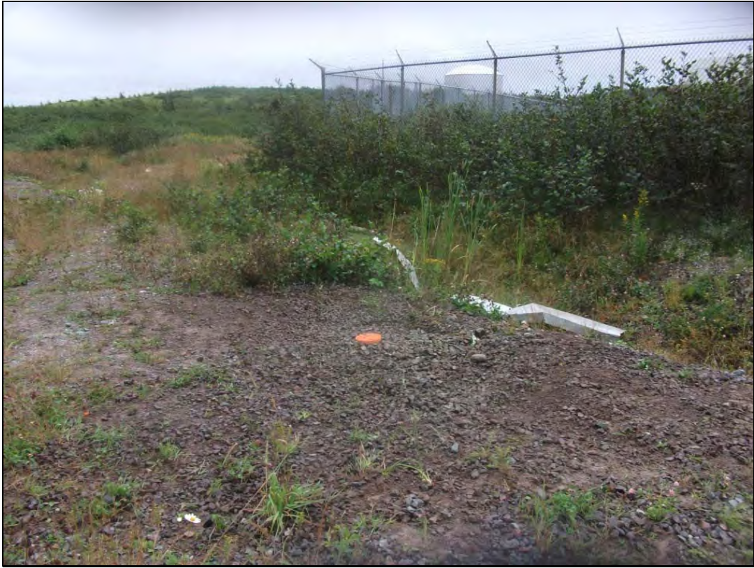
Photo 9: View, looking northeast, showing Clean-out 2 after modifications (typical) with painted flushmount cover.
