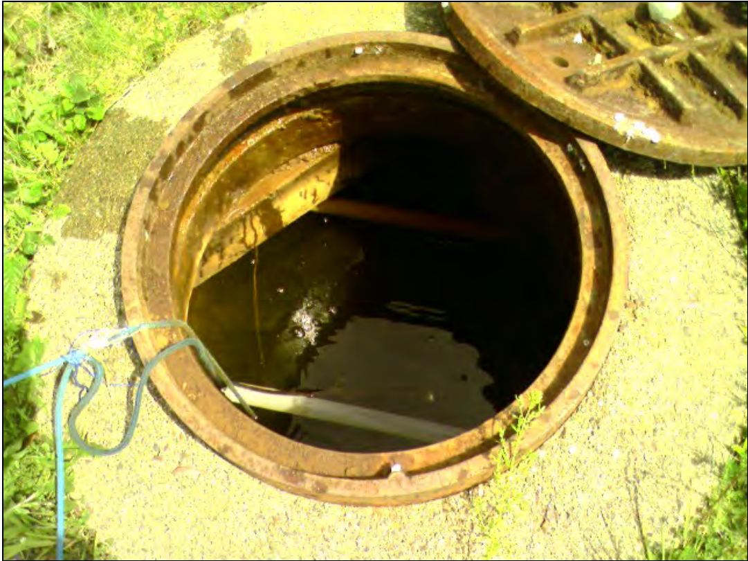
Photo 3: View of PLCS valve chamber prior to July 2010 sampling event. Note discharge hose floating in the chamber (upper corner).
