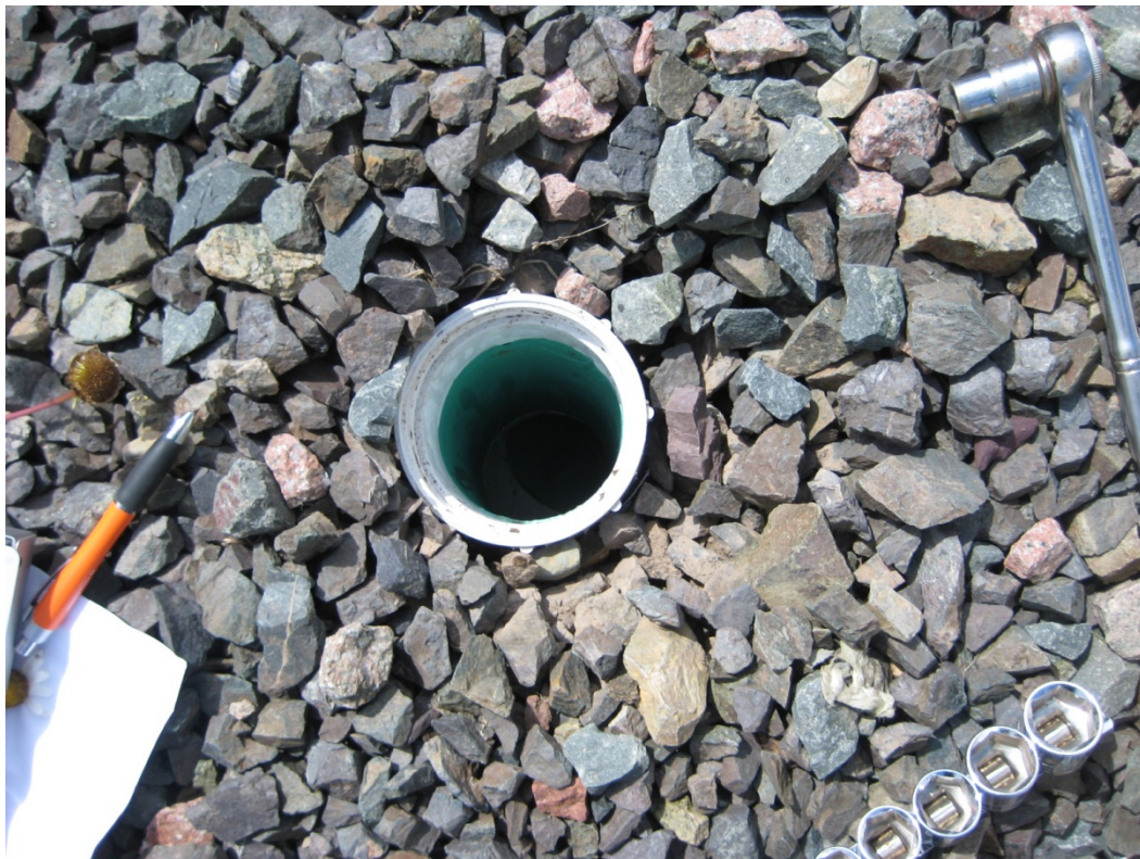
Photo 2: View of groundwater drainage system clean-out pipe (CO3).
