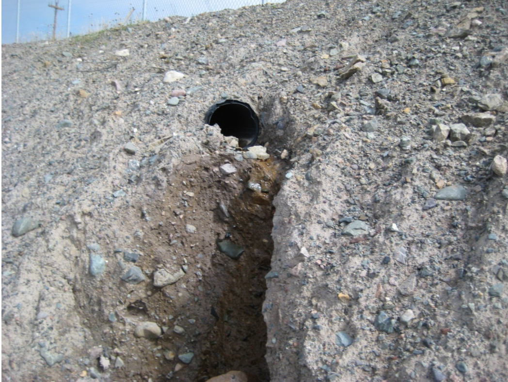
Photo 3: View of groundwater drainage system outflow drainage pipe. Note: the pipe has been cut off and the grate removed.
