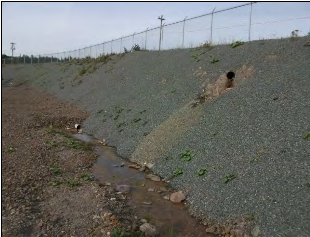
Photo 4: View, looking northeast, of new discharge location of groundwater interception system during the August 2012 Site visit, which is located within the boundaries of the newly constructed asphalt plant. Note discharge pipe without a rodent screen.
