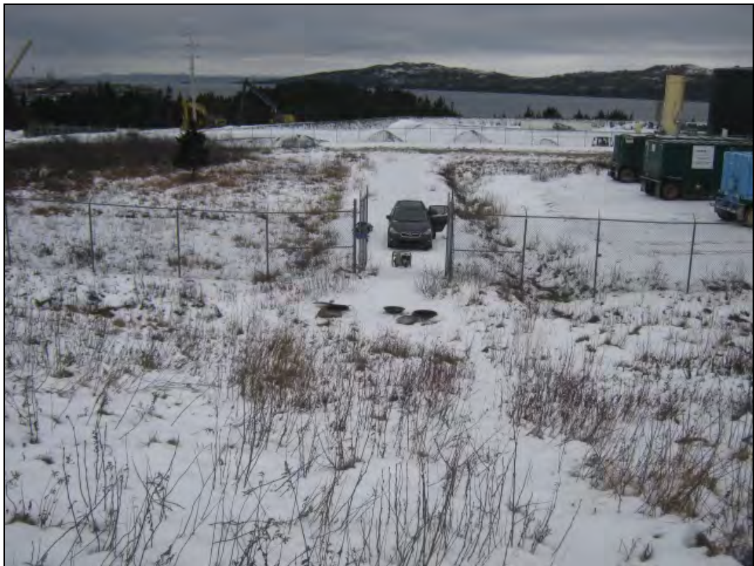
Photo 8: View, looking west, while preparing for the December 2012 pump down test of the SLCS valve chamber.
