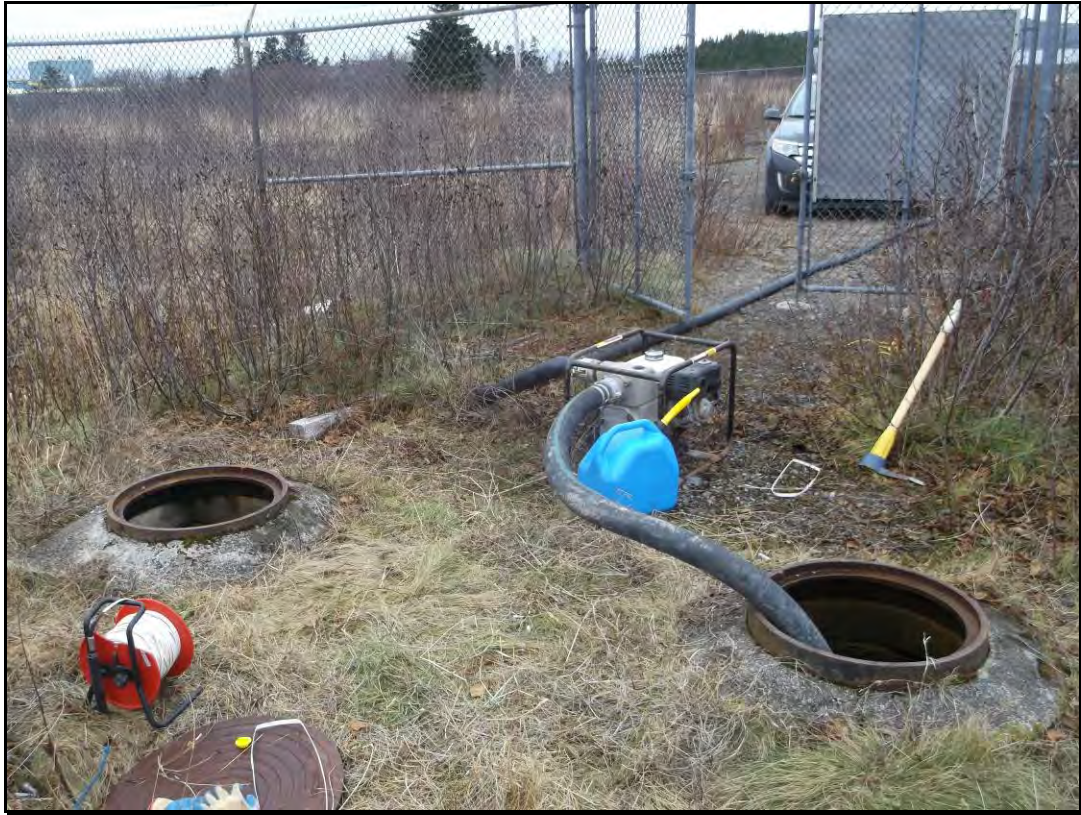
Photo 11: View, looking southwest, while pumping leachate from the PLCS and SLCS valve chambers in December 2014.
