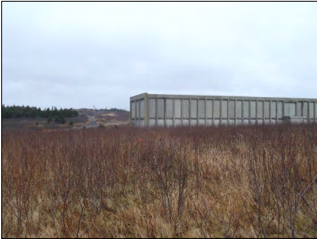
Photo 7: View, looking northeast, showing the vegetative overgrowth at the ECP-1 during the landfill cover inspection in December 2014.
