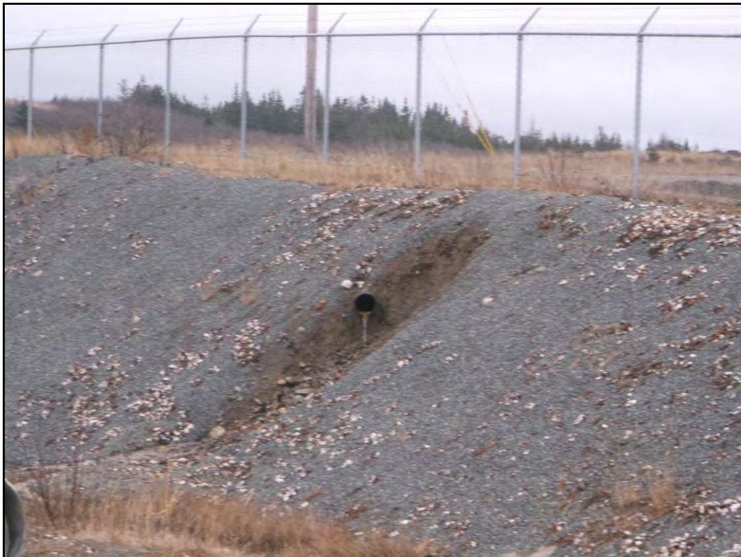
Photo 10: View, looking northeast, showing the groundwater interception drainage system during the November 2014 site visit. Note discharge pipe without a rodent screen and iron oxide staining.
