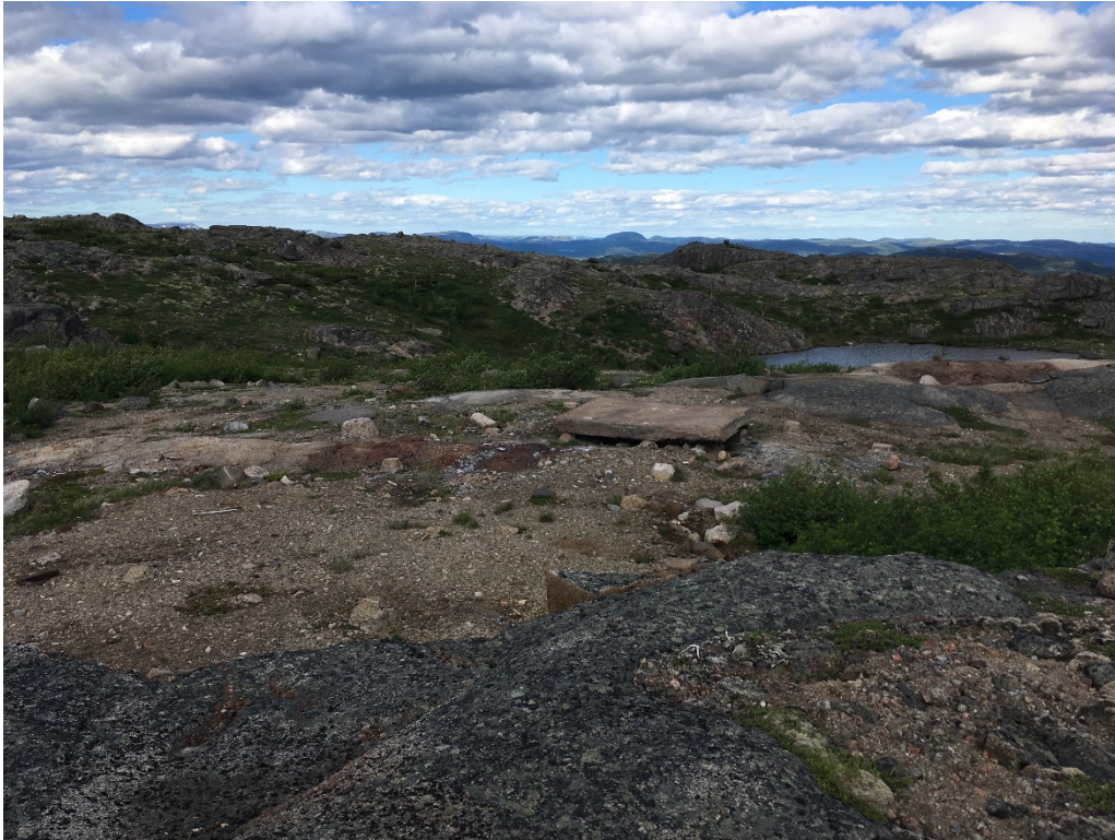
Photo 1 Upper Site: concrete pad and foundation of former site structure. Looking north.
