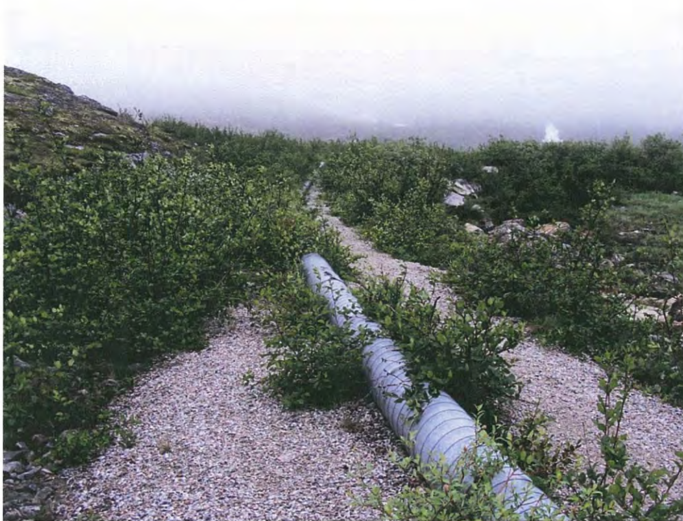
Photo 6 View of water line from the Reservoir
