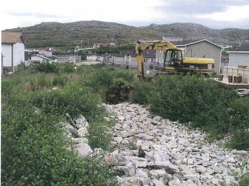
Photo 7 View of debris cleanup in the stream northeast of the Residential Subdivision
