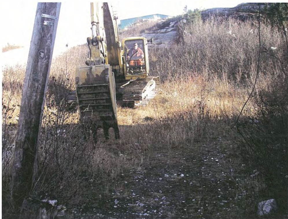
Photo 10 View of excavator preparing to dig a test pit in the Residential Subdivision
