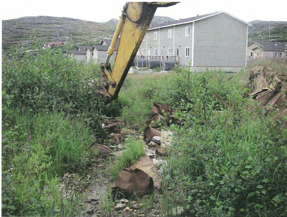
Photo 6 View of debris cleanup in the stream northeast of the Residential Subdivision
