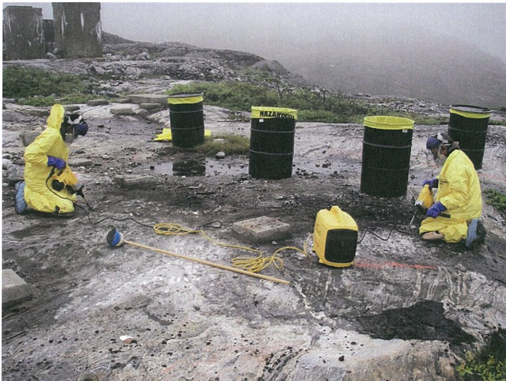
Photo 6 Limited remediation of PCB-impacted tar at Old Base 1
