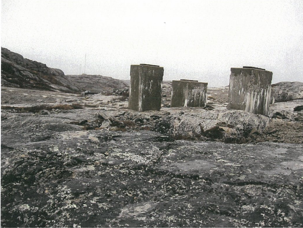
Photo 3 Concrete foundations at the Old Base 1 site (looking east). The black truck in the background is parked on the main access road.
