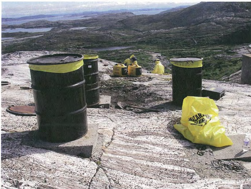
Photo 14 View of limited remediation of PCB-impacted tar at the Main Base site
