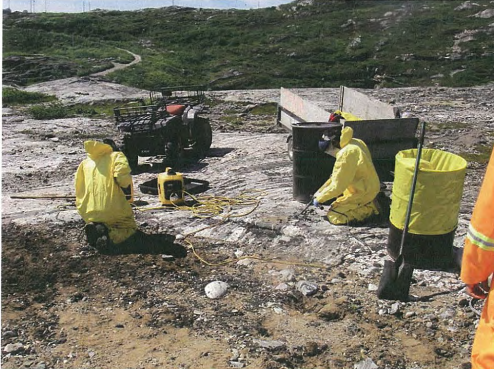
Photo 13 View of limited remediation of PCB-impacted tar at the Main Base site
