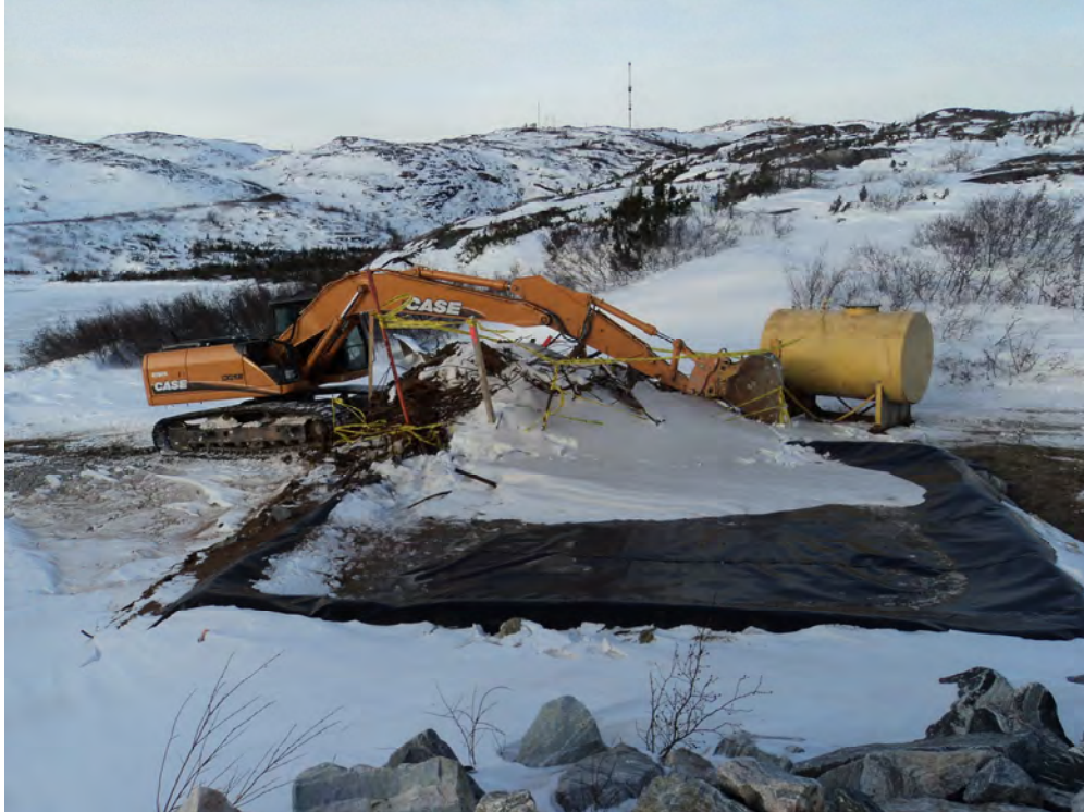
Photo 17 View of scrap metal covered with excavator bucket at the Old Dump Pond site on December 15, 2011.
