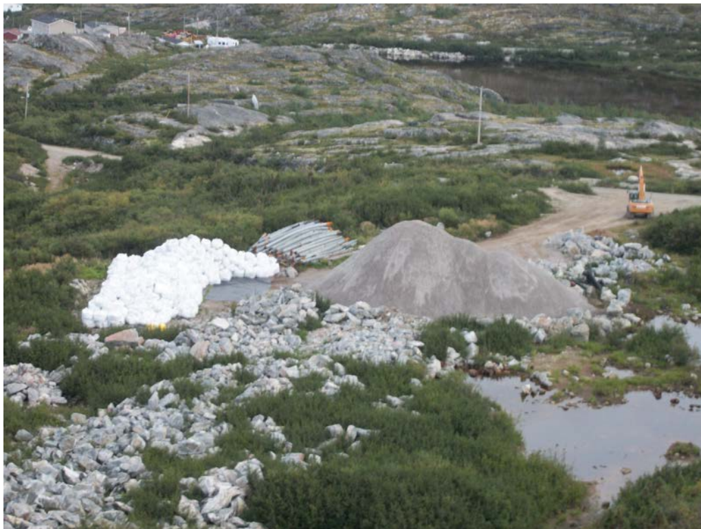
Photo 24 Laydown area and stockpiled backfill material at Pit No. 1 on August 25, 2012, looking southeast.
