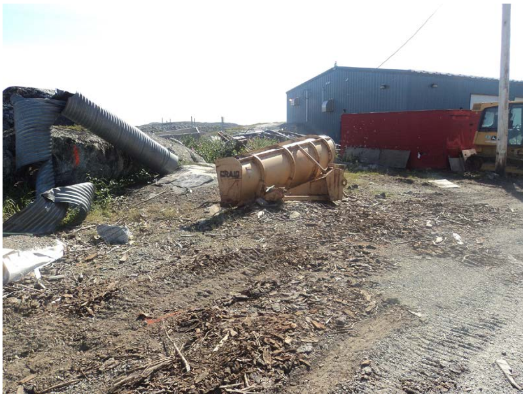
Photo 18 Area south of the road at the Wharf site prior to soil removal.
