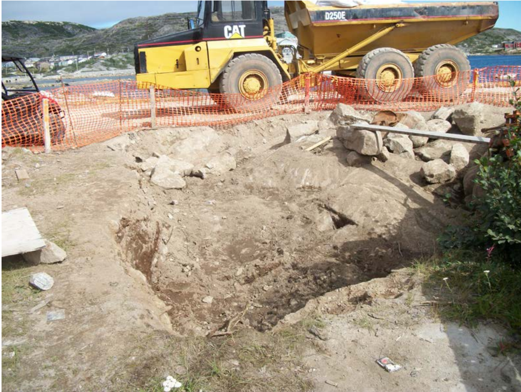
Photo 19 Area south of the road at the Wharf site during soil removal.
