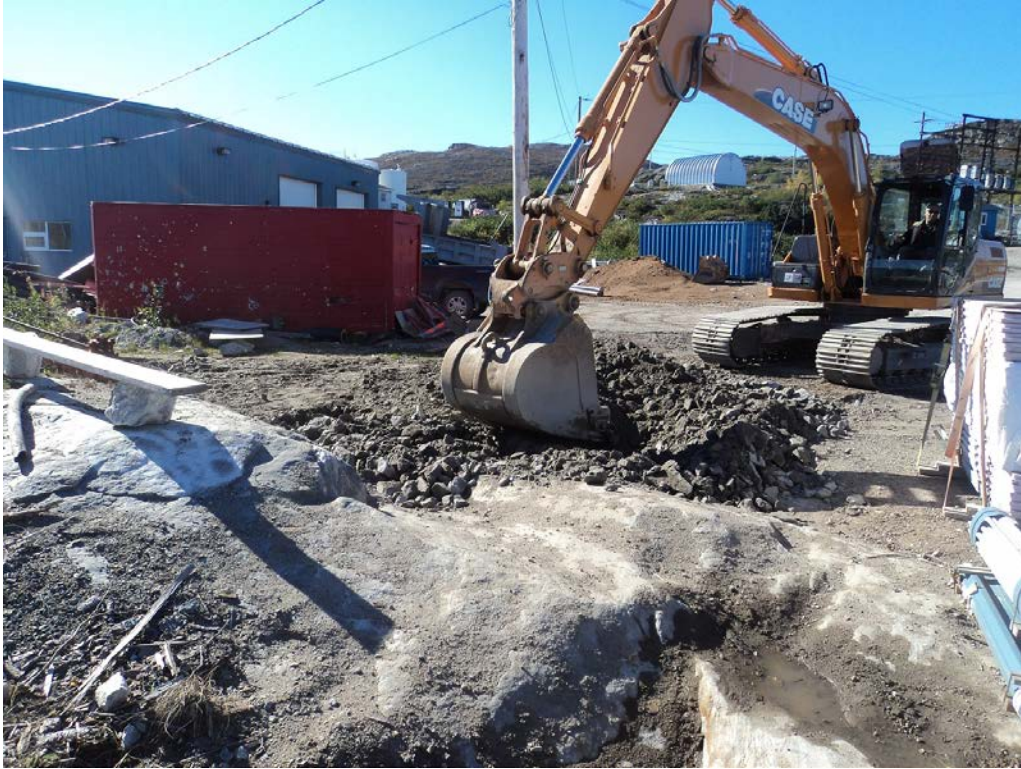
Photo 21 Backfilling of area south of the road at the Wharf site on September 18, 2012.
