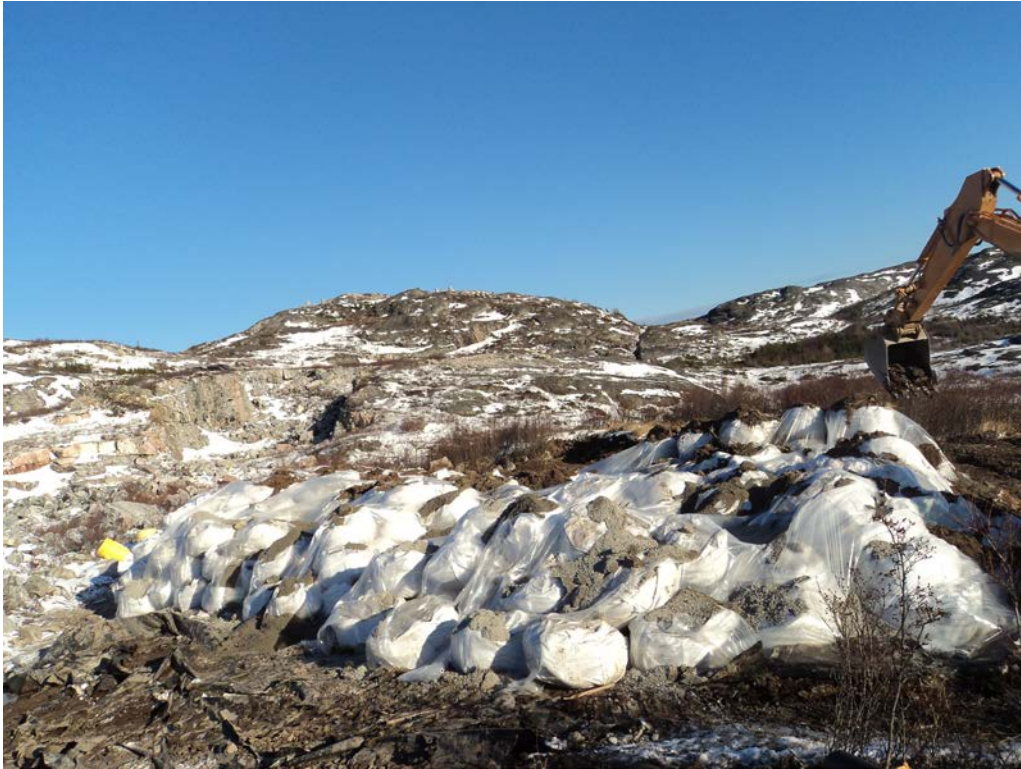
Photo 29 Bags remaining at laydown area following barge loading (bags covered in plastic).
