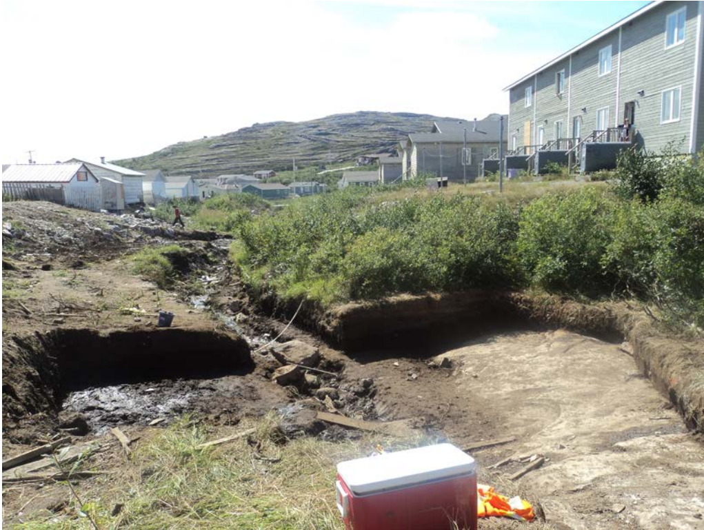
Photo 11 Upper portion of the stream on August 14, 2012 (looking south), following additional soil removal.
