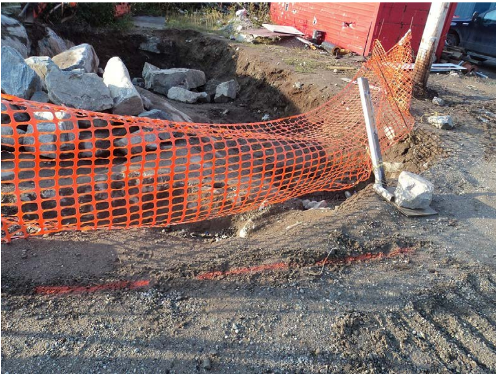
Photo 20 Area south of the road at the Wharf site during soil removal (terminated on bedrock).
