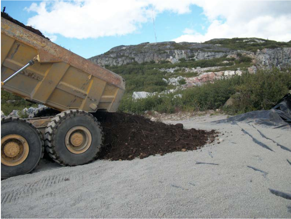
Photo 48 PCB-impacted soil in the Staging Area.
