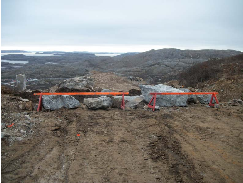
Photo 33 Boulders and barricades placed along the northeast limits of the Main Base-Area 1 excavation.
