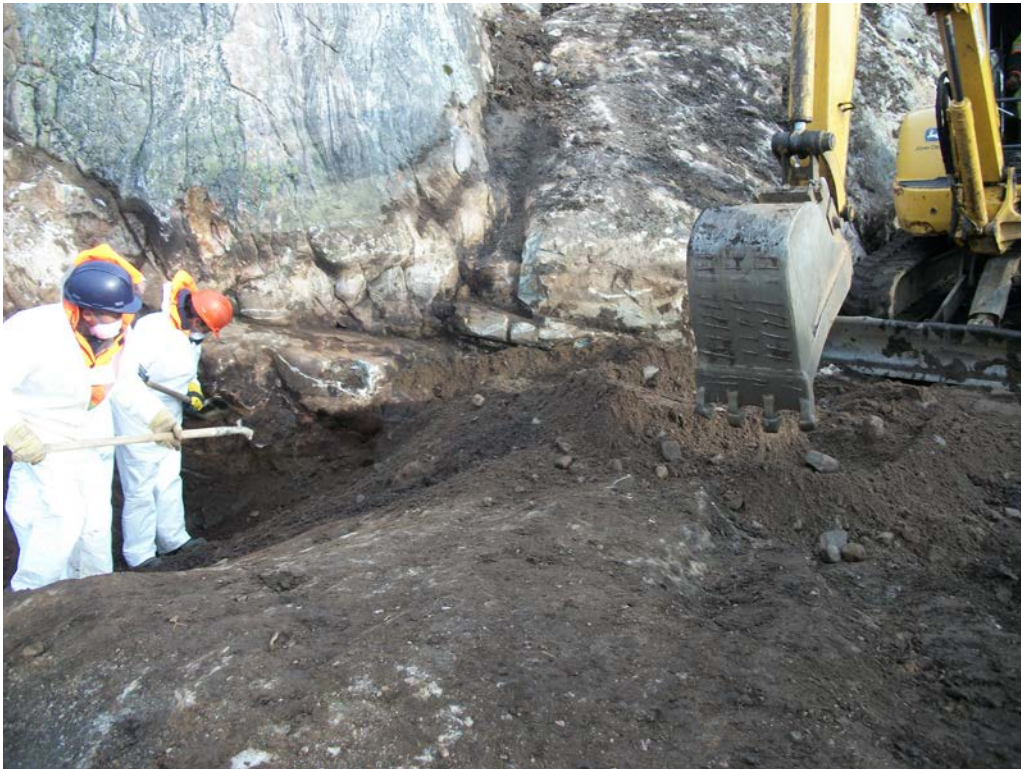
Photo 30 Removal of PCB-impacted soil and tar-like material in the vicinity of former sample 22488 at Main Base-Area 1.
