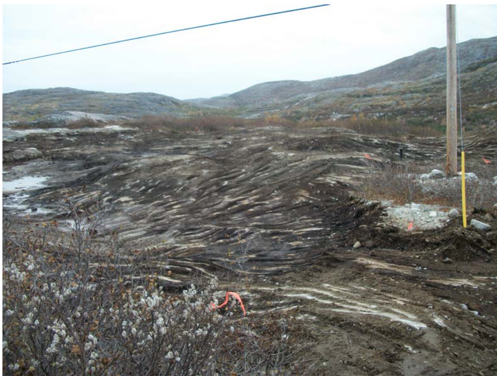
Photo 40 TPH-impacted soil removal at POL Compound (note: remaining soil on bedrock was manually removed using shovels).
