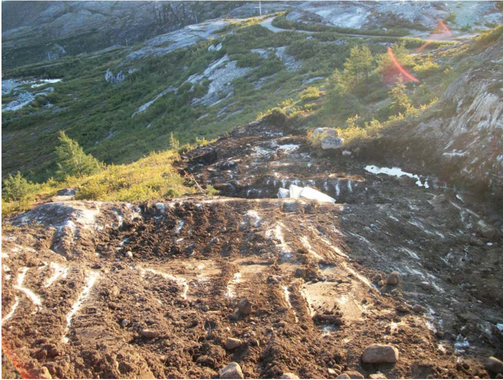
Photo 35 TPH-impacted soil removal at Main Base-Area 7 (note: remaining soil on bedrock was manually removed using shovels).
