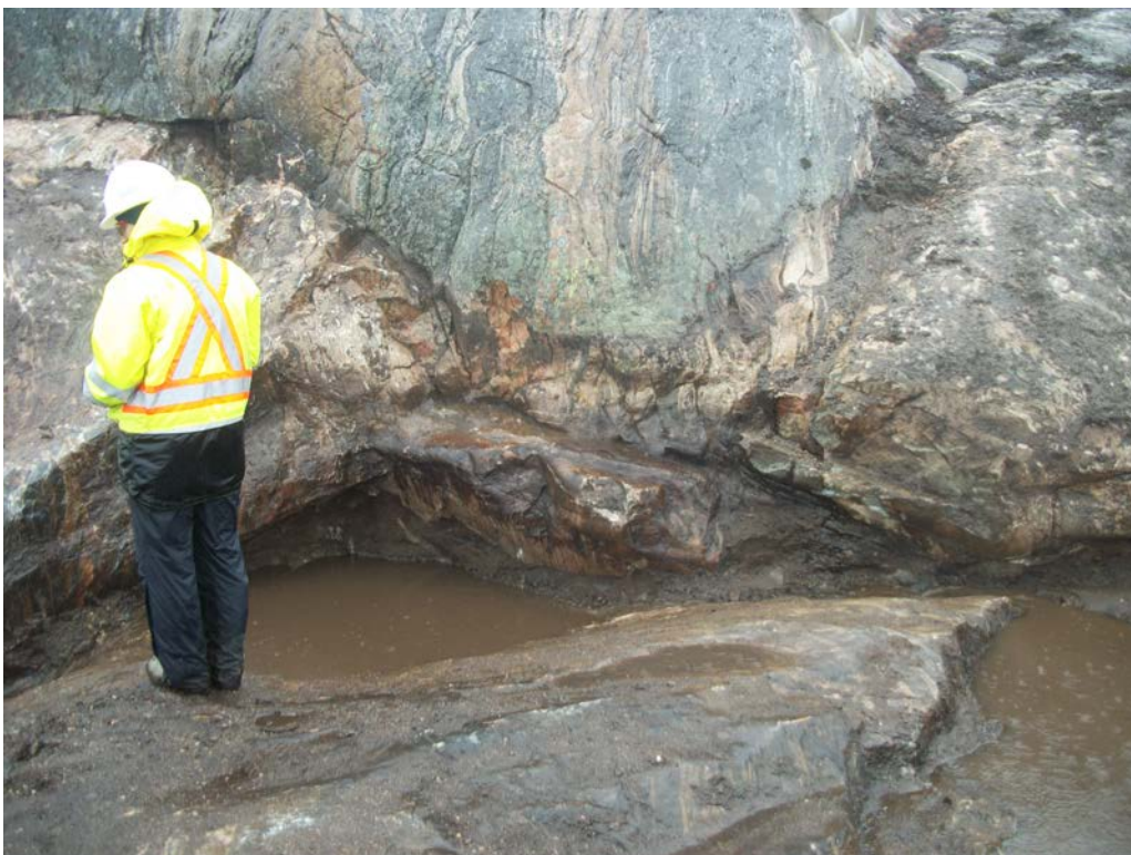
Photo 32 Main Base-Area 1 following the removal of PCB-impacted soil and tar-like material in the vicinity of former sample 22488.
