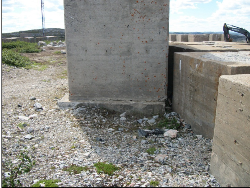
Photo 9. Area of cadmium-impacted soil requiring remediation (BS7), looking west.
