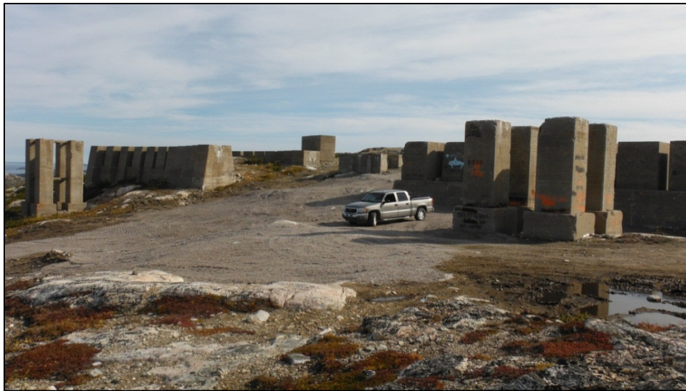
Photo 2. 2013 photo of BMEWS following the removal of PCB-impacted soil and site-reinstatement, looking southeast (remediated area is backfilled with clean material).
