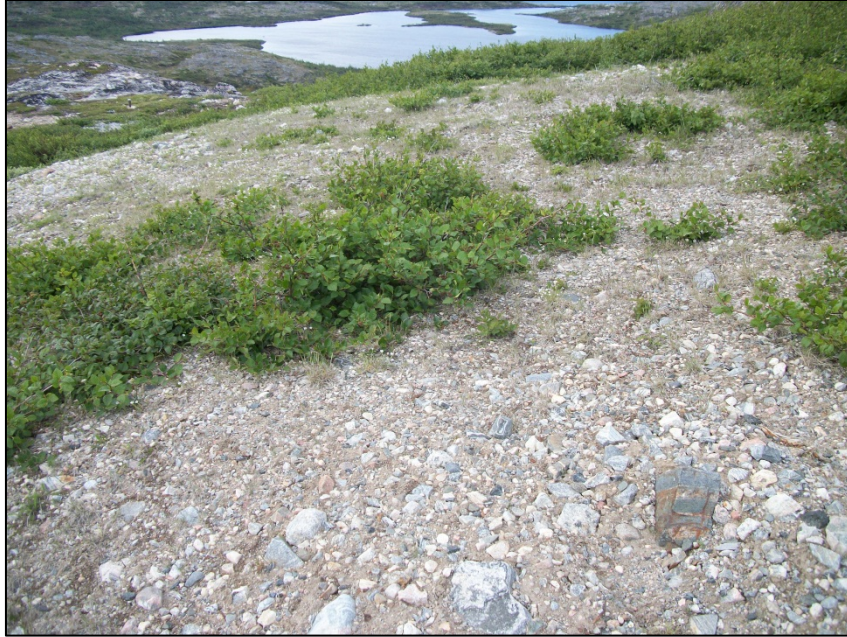
Photo 5. Area of TPH-impacted soil requiring removal (and TP-102 and BMEWS-TP11), looking northwest.
