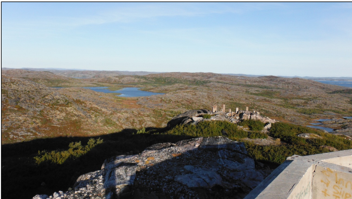
Photo 4. Concrete foundations currently remaining at Main Base, looking northwest towards Big Lake
