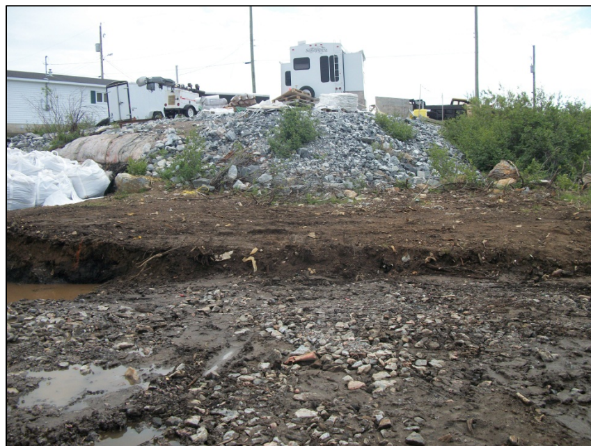
Photo 4. Approximate location of metals (antimony) impacted soil requiring remediation at depth (TP-233), looking east.
