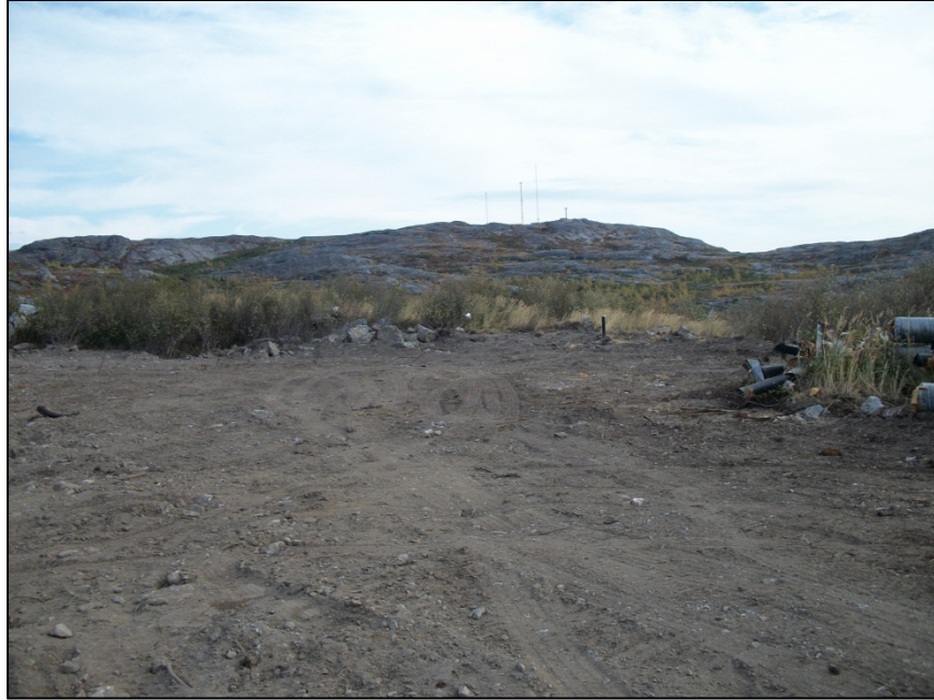
Photo 1. Pit No. 1 in 2011 prior to the installation of liners for temporary soil storage, looking northeast.
