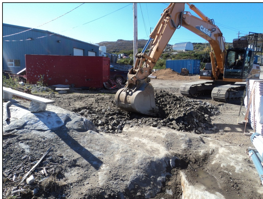
Photo 4. Area south of the road at the Pipeline/Wharf area during site reinstatement in 2012.
