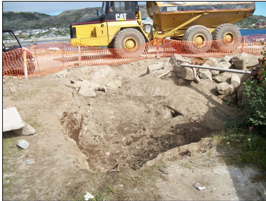
Photo 3. Area south of the road at the Pipeline/Wharf area during soil removal in 2012.
