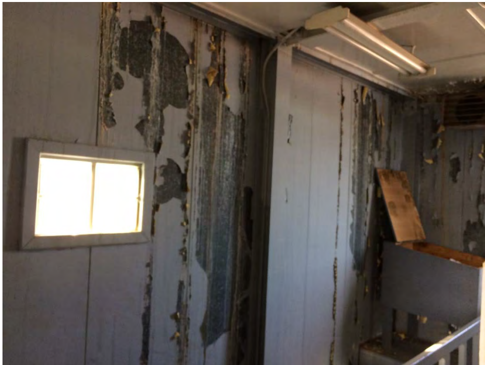
Photo 18: Syncrolift Building – Second Floor where peeling grey over green over yellow paint was confirmed to be above Human Health criterion and below TDG criterion. Vinyl floor tile and mastic were confirmed as ACM.
