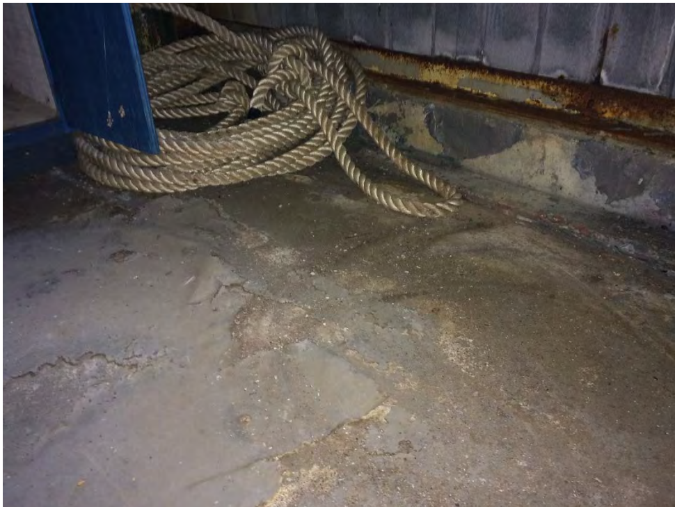
Photo 22: Services Building – Rigger's Room back area where peeling grey paint on the concrete floor and curb was confirmed as lead-based. Potential ACMs were not observed.
