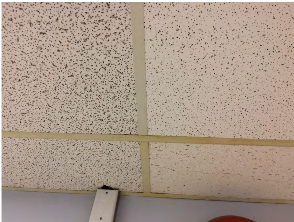
Photo 28: Administration Building – Second Floor Gym area where three types of ceiling tile confirmed as no ACMs.
