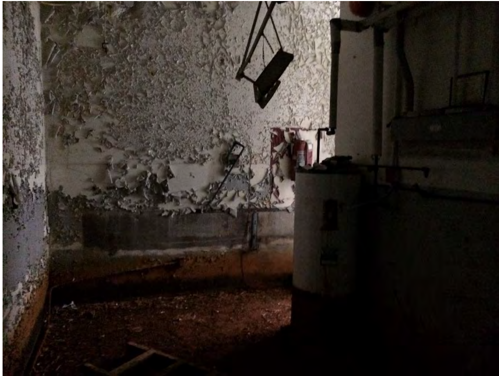
Photo 35: Administration Building – Mechanical Room where peeling and flaking grey paint on lower wall with peeling and flaking white paint on upper wall ceiling that confirmed lead concentrations above the Human Health criterion.
