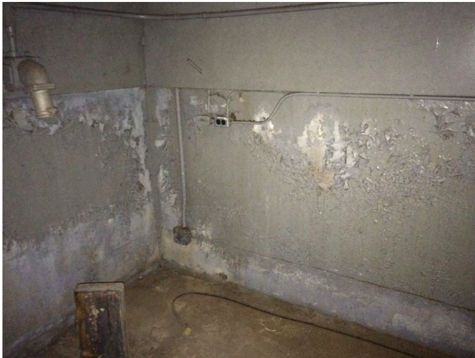
Photo 12: Assembly & Erection Building – Sheet Metal Shop walls where grey paint was confirmed to be above Human Health criterion and below TDG criterion.
