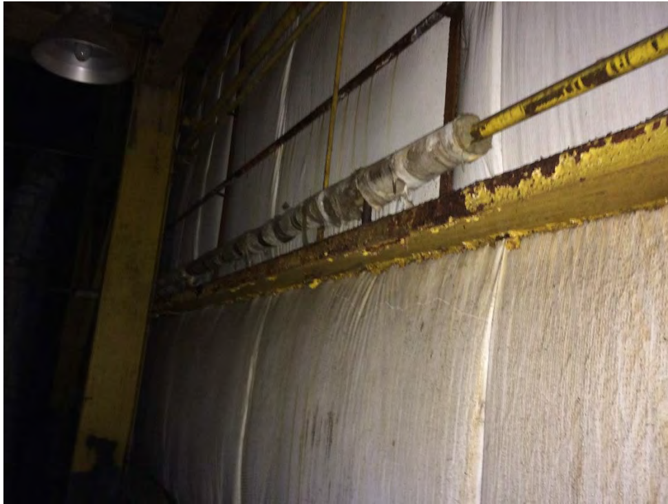
Photo 15: Assembly & Erection Building – Structural steel with occasional areas of peeling yellow paint confirmed to be lead-based. Also note ACM pipe insulation in poor condition.
