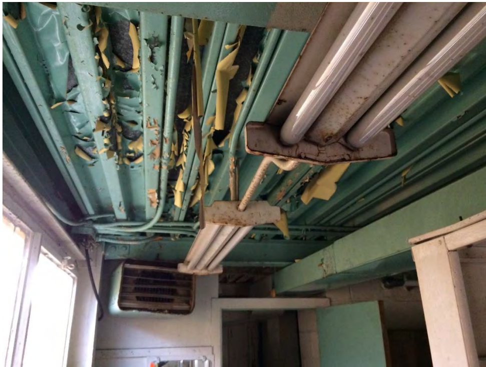
Photo 17: Syncrolift Building – Main Floor where peeling teal green over yellow paint was confirmed to be lead-based. ACM pipe insulation was not observed in the ceiling space.
