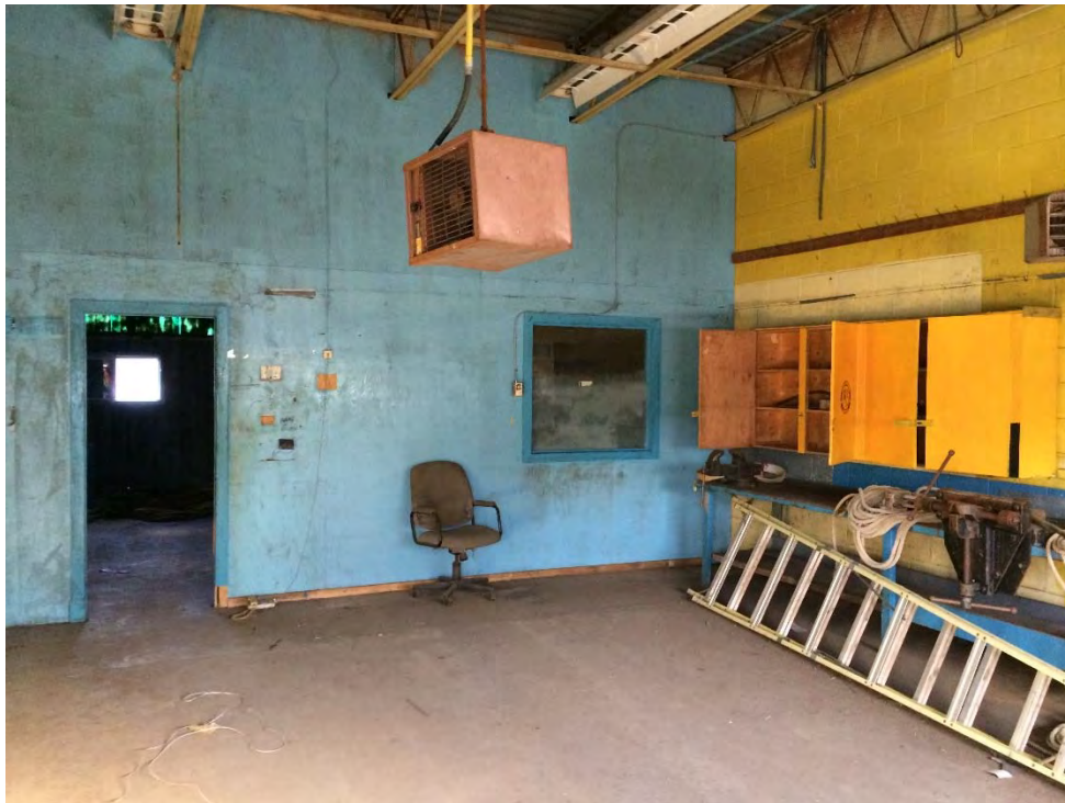
Photo 21: Services Building – Rigger's Room where flaking or peeling paint or potential ACMs were not observed.
