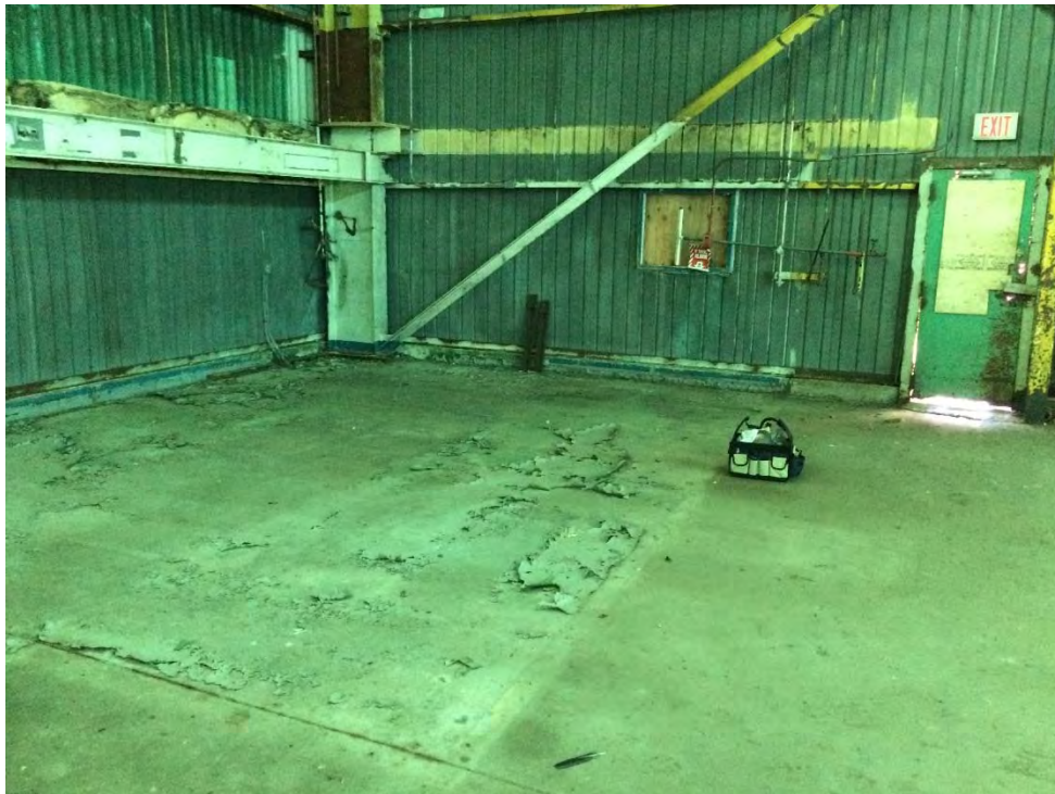
Photo 4: Carpenters & Joiners Building – Main Floor front corner of Machine Shop area where grey over green peeling lead-based paint was confirmed
