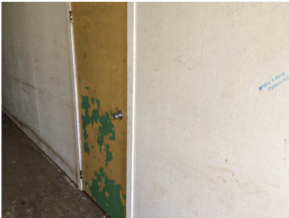
Photo 36: Murley Building – Second Floor storage room door with peeling and flaking yellow over green paint that was confirmed as lead-based. Small quantities of flaking paint were observed on the floor in the hallway.
