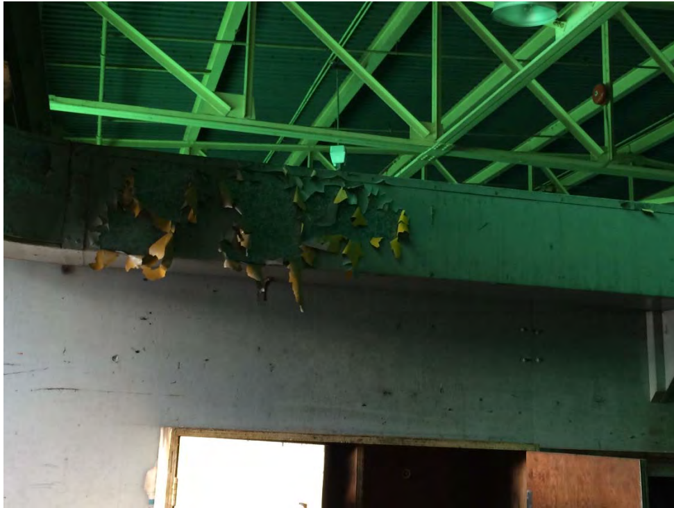
Photo 5: Carpenters & Joiners Building – Second Floor Dry Stores area where peeling green over yellow lead-based paint was confirmed .
