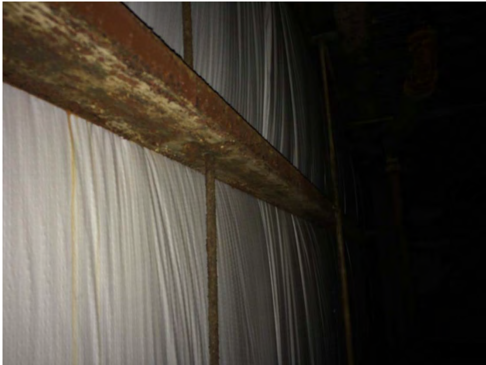
Photo 16: Assembly & Erection Building – Wheelabrator equipment area where small flaking was observed of black over cream over green paint was confirmed as lead-based.
