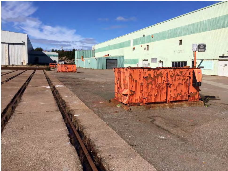
Photo 38: Docking Berths & Side Transfer Area – Steel electrical containment boxes with heavy corrosion and flaking orange paint that was confirmed as lead-based.
