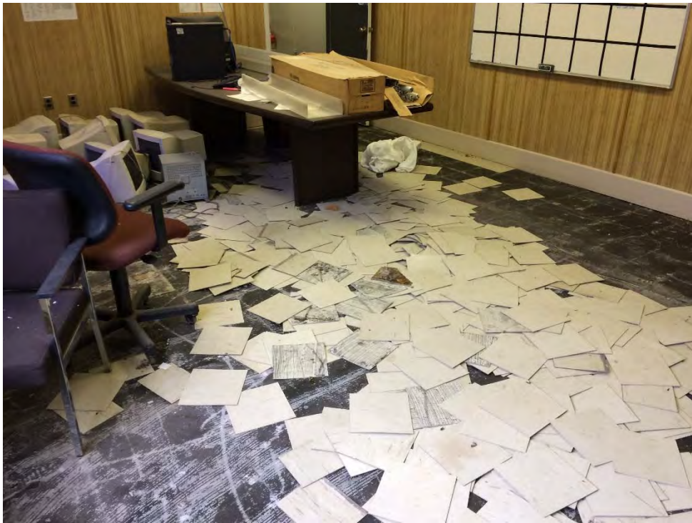
Photo 31: Administration Building – Main Floor Board Room (former Accounting Machines) where the light brown vinyl floor tile and mastic was confirmed ACMs . Accessible pipe insulation was previously removed from the ceiling space.
