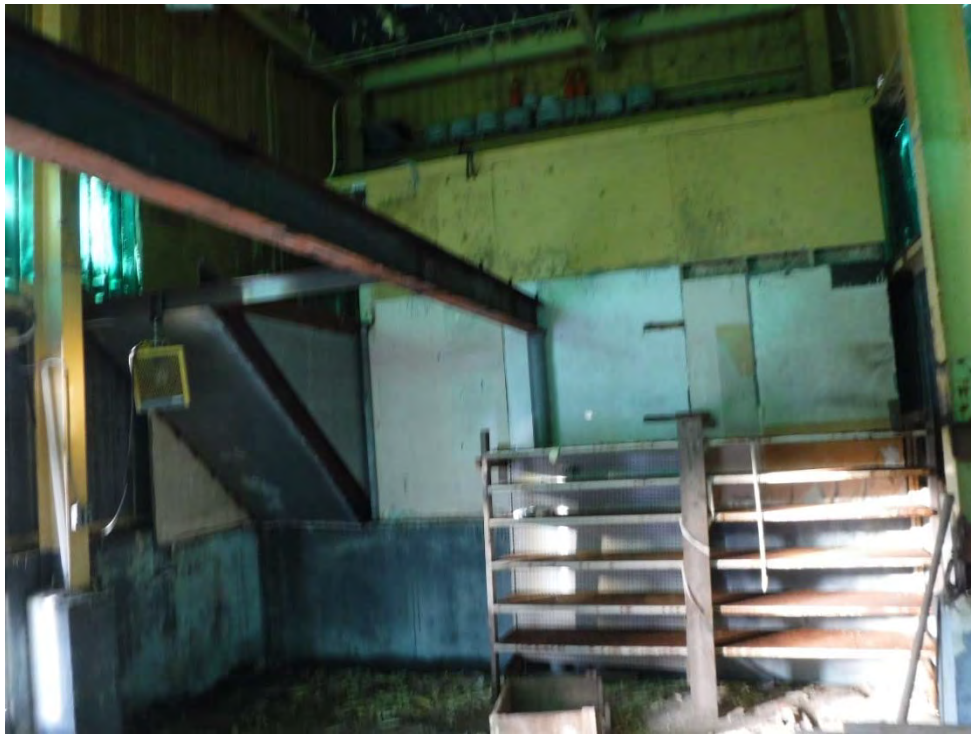
Photo 25: Parts Building – Loading bay where peeling yellow over cream paint was confirmed as lead-based. Paint flakes were noted to cover the floor area and potential ACMs were not observed.
