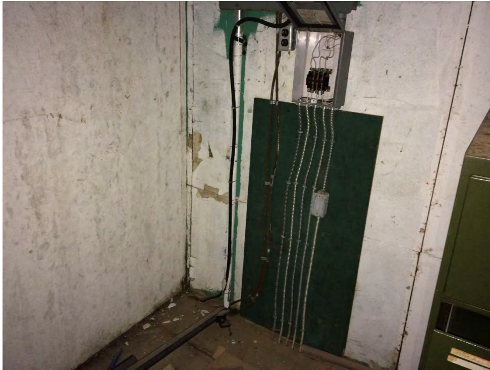
Photo 37: Murley Building – Second Floor storage room wall with flaking and peeling white paint that confirmed lead concentrations above the Human Health criterion. Some flaking paint was observed on the floor and cabinets.
