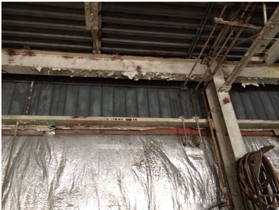
Photo 24: Services Building – Garage where white over yellow peeling paint was confirmed as lead-based; flakes were also observed on the floor. Potential ACMs were not observed.
