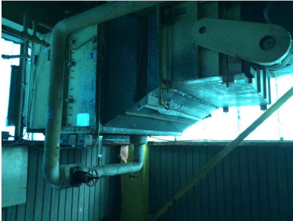
Photo 1: Carpenters & Joiners Building – Main Floor heating unit pipe elbow insulation confirmed as ACM.
