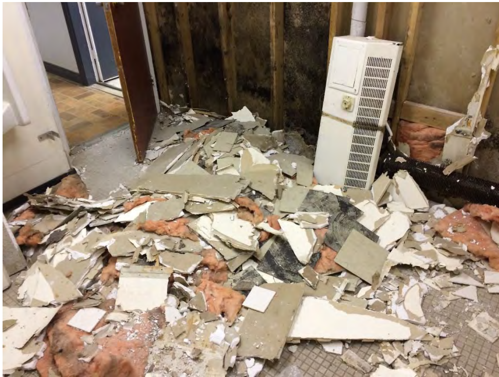
Photo 33: Administration Building – Main Floor Washroom where accessible ACM pipe insulation was previously removed. Note remaining debris following a water leak repair, but mould impacted surface remains in drywall.
