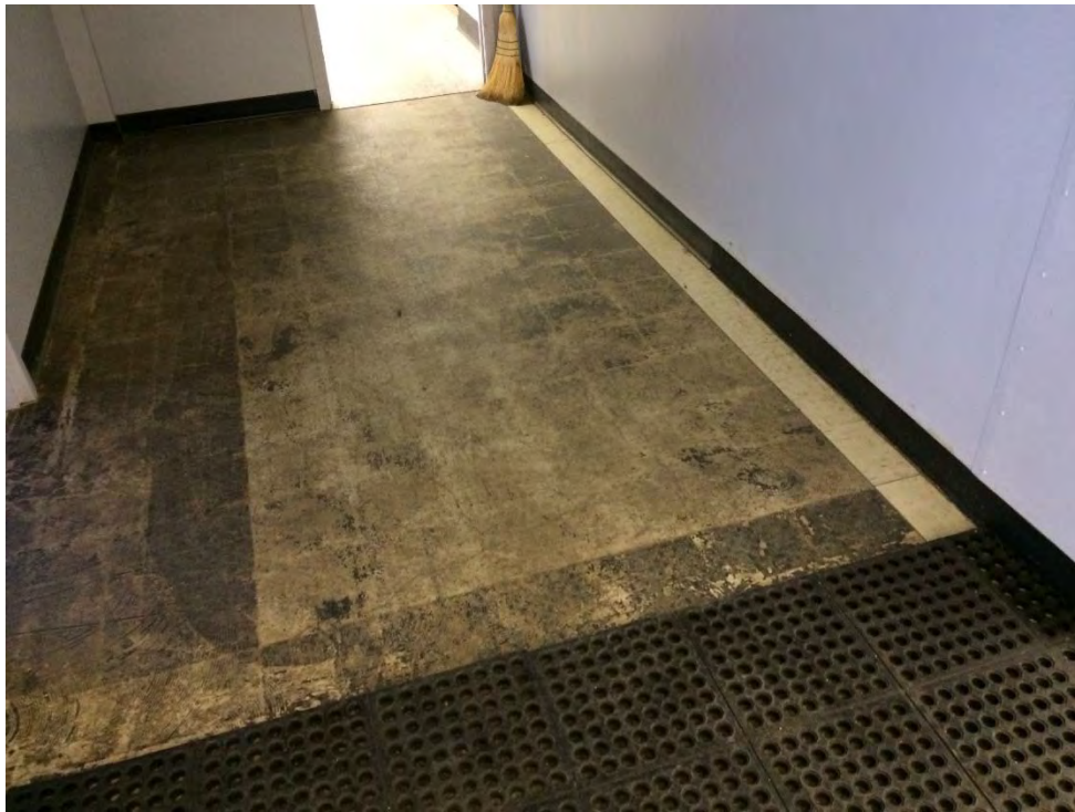
Photo 27: Administration Building – Second Floor hall by centre stairwell where remaining vinyl floor tile and mastic confirmed as ACM.
