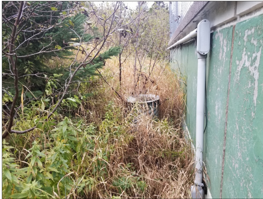
Photo 9 – View, looking west, of RW2 along the south side of the Main Administration and Security Office (MASO).
