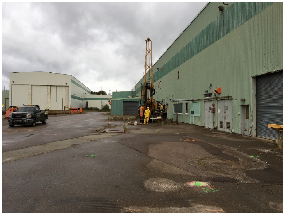
Photo 21 – View, looking northwest, of the Marystown Shipyard General Stores Building (MSGB), while drilling MSGB-BH1-2018.
