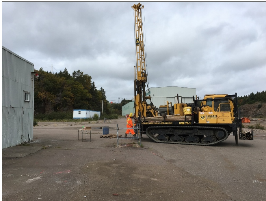
Photo 19 – View, looking south, of the Marystown Shipyard Service Building (MSBL), while drilling MSBL-BH1-2018.
