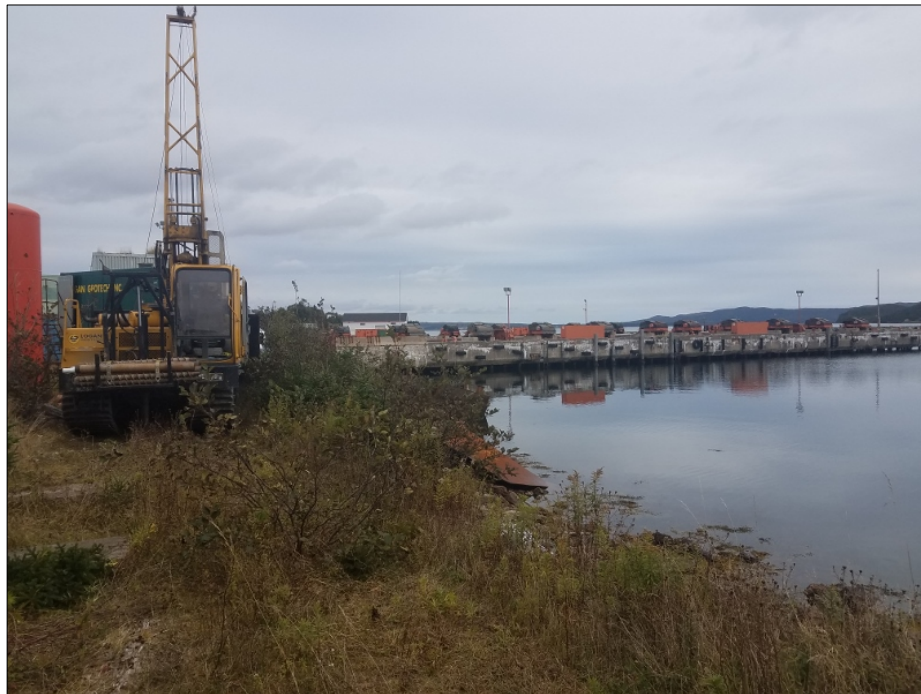
Photo 20 – View, looking northeast, while drilling MSBL-MW2-2018 in the Marystown Shipyard Service Building (MBSL) area. Note the waterlot to the right of the photograph.
