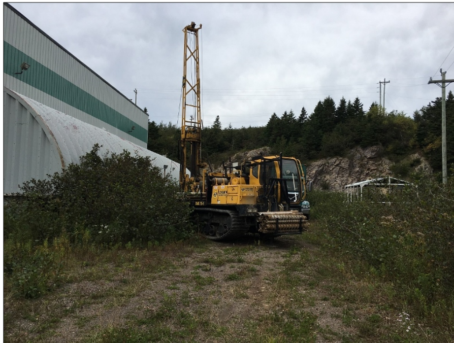
Photo 10 – View, looking southwest, of the Marystown Shipyard Assembly and Erection Building (MAEB) while drilling MAEB-MW2-2018.
