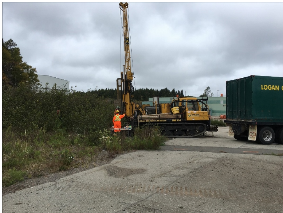
Photo 12 – View, looking north, of the Marystown Shipyard Fuel Pump Area (MFPA), while drilling MFPA-BH2-2018.
