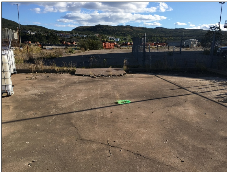
Photo 2 – View, looking southwest, of the Marystown Shipyard Drum Storage Area (MDSA) with existing monitor well MDSA-MW9 in the foreground.
