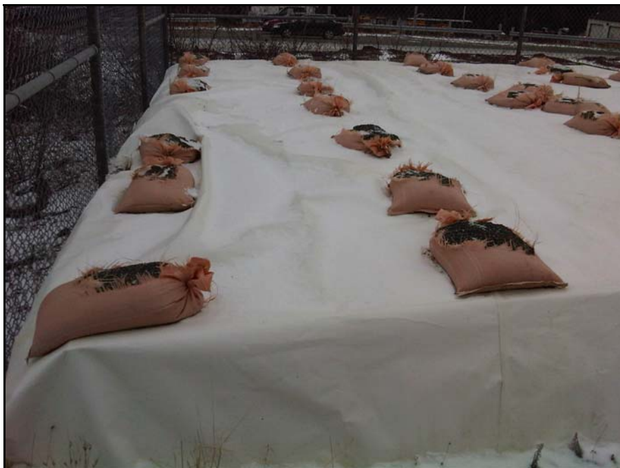
Photo 16: Weathered sand bags.
