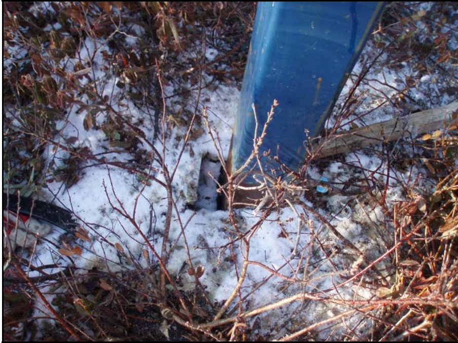
Photo 3: MW-07 base separated from grout.
