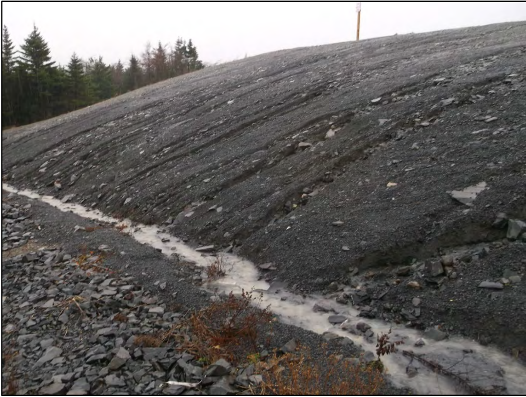
Photo 11: View, looking southwest, toward the existing waste disposal site. Note the erosion on the landfill cover.
