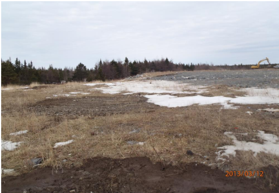
3. Looking northeast at the PCB Area and former TP locations (exposed soil).
