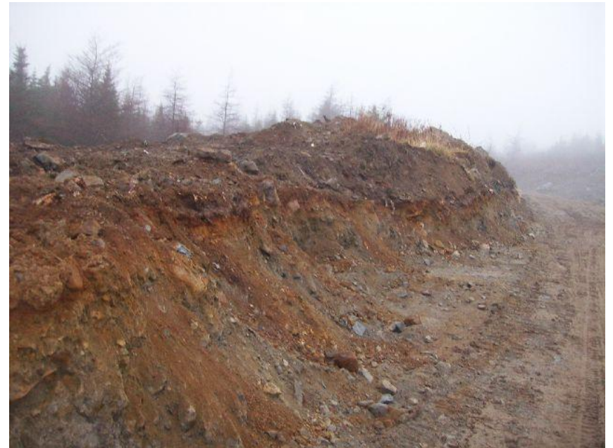
Photo 24 – Excavated site access road showing thin layer of waste (Dec 6)
