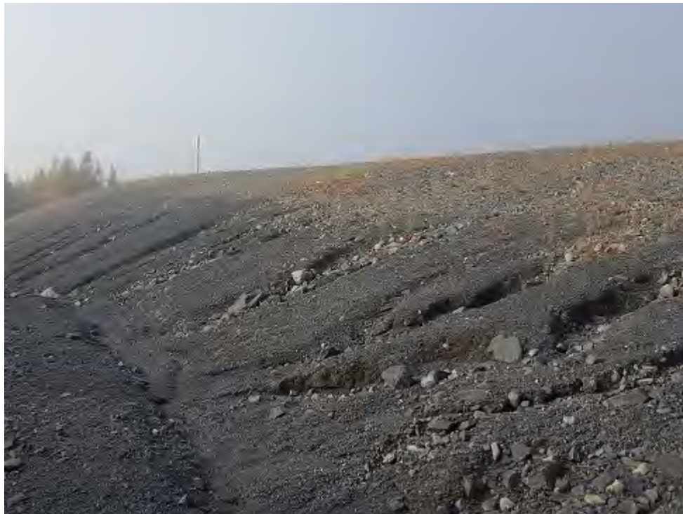
Photo 10 - View of the waste disposal slope looking southeast showing erosion of the landfill cover.
