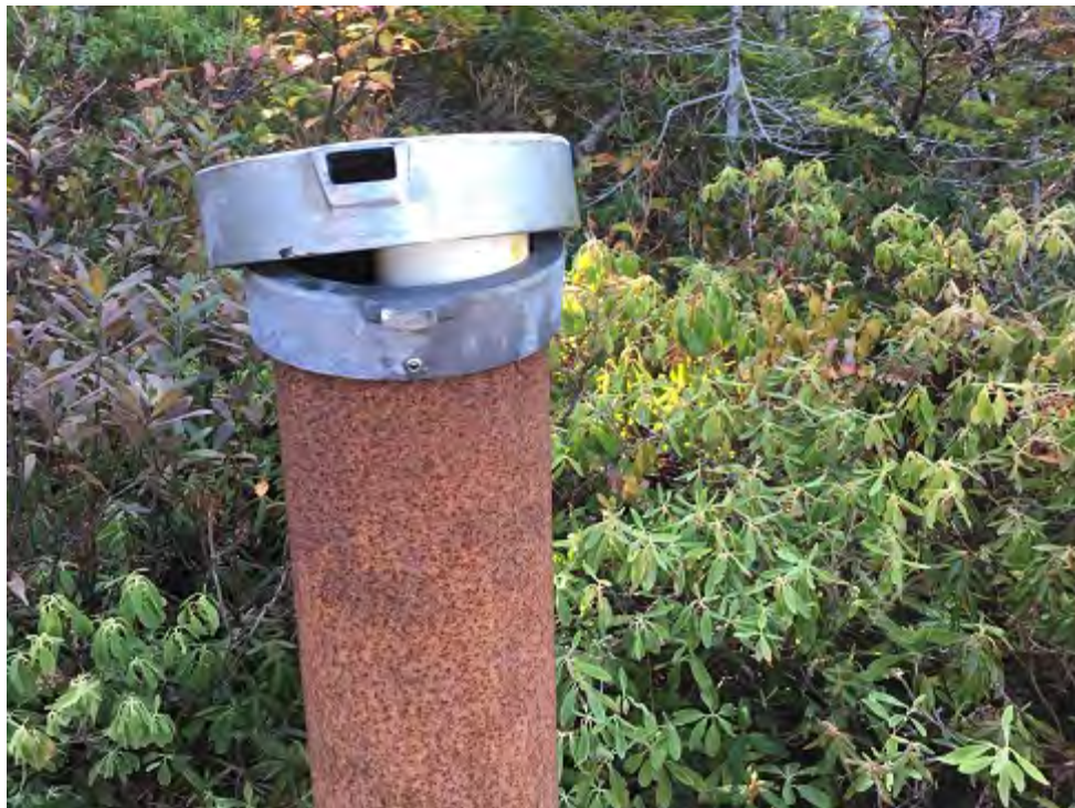
Photo 4 - View of MW-08 facing south during the October 2017 monitoring event. Note the well cap does not fit over the PVC casing stick up.
