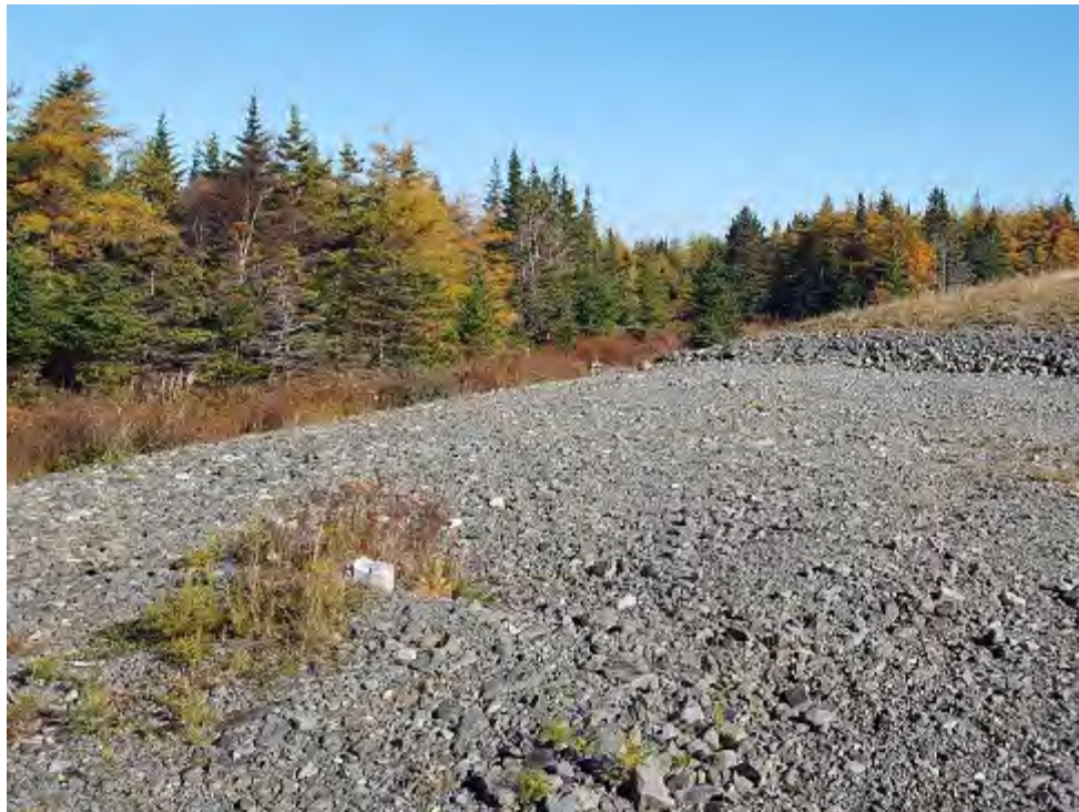
Photo 9 - View of missing No Trespassing/No Dumping sign on southwest corner of the landfill cover.
