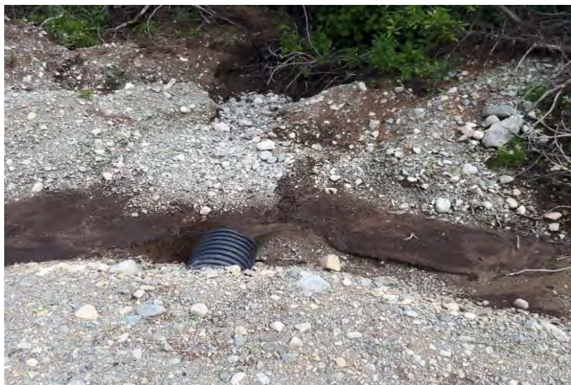
Figure 41: Muir Creek Discharging into Roadside Ditch
