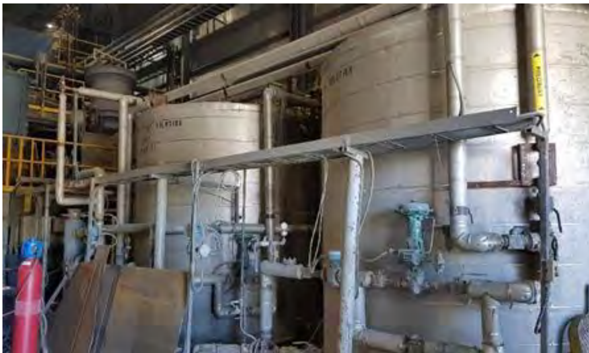
Figure 17: Existing Gold Circuit at Nugget Pond Mill
