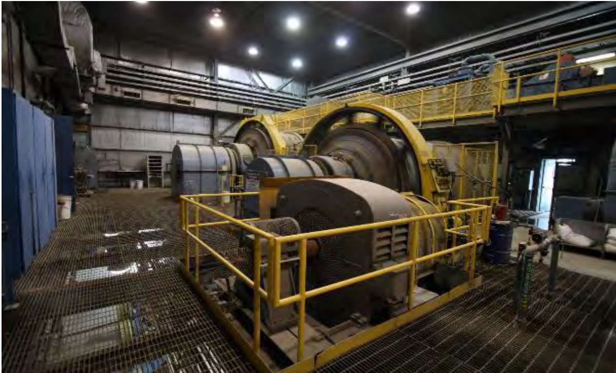
Figure 18: Existing Grinding Mill at the Nugget Pond Mill
