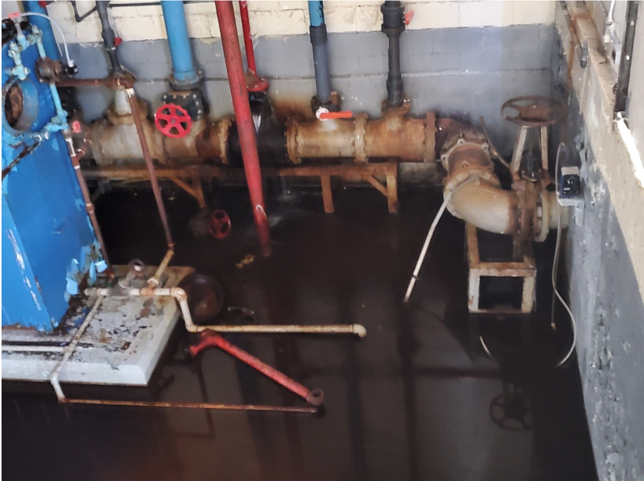
Figure 71 - Charleston Plant Flooding
