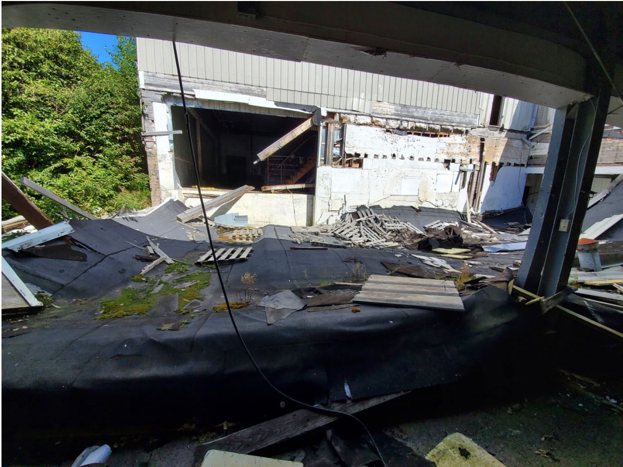
Figure 72 - Charleston - Roof Collapse 1
