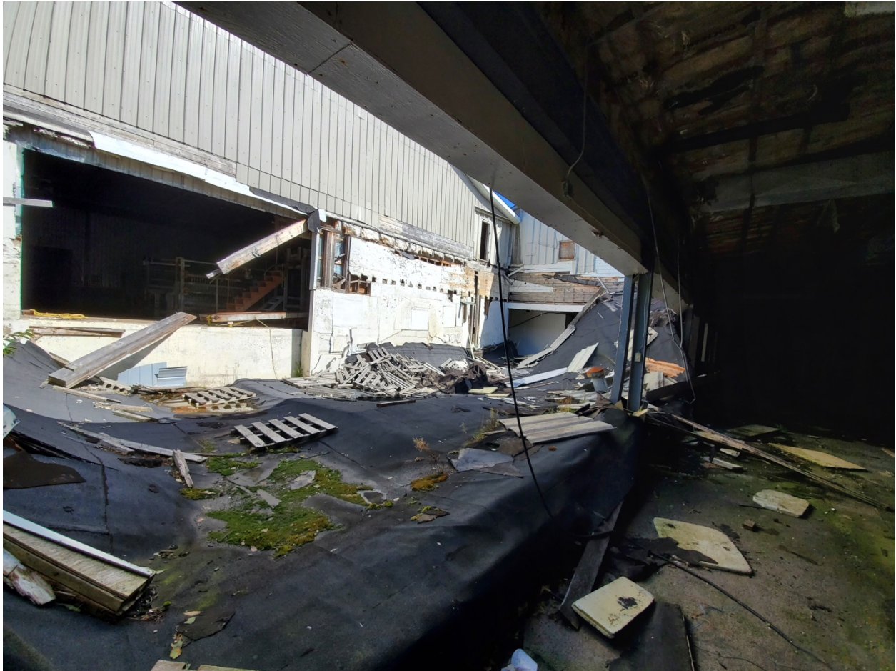
Figure 73 - Charleston - Roof Collapse 2
