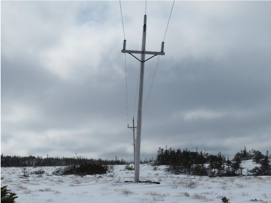
Figure A-5: Leaning Pole missing Crib
