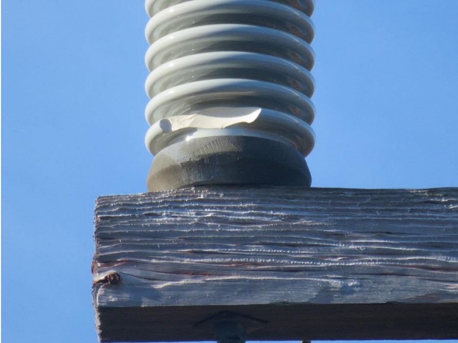
Figure A-4: Chipped Porcelain Insulator
