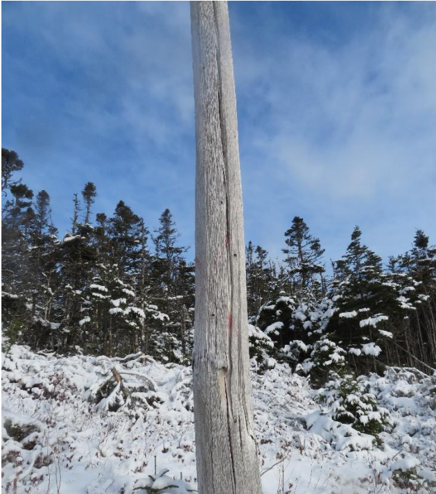
Figure 3 Deteriorated pole with horizontal split
