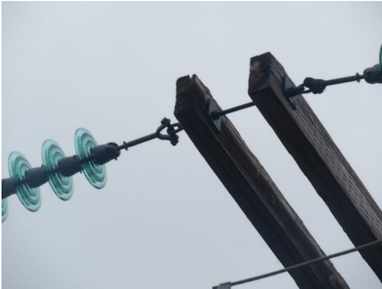
Figure A-1 Split Crossarm
