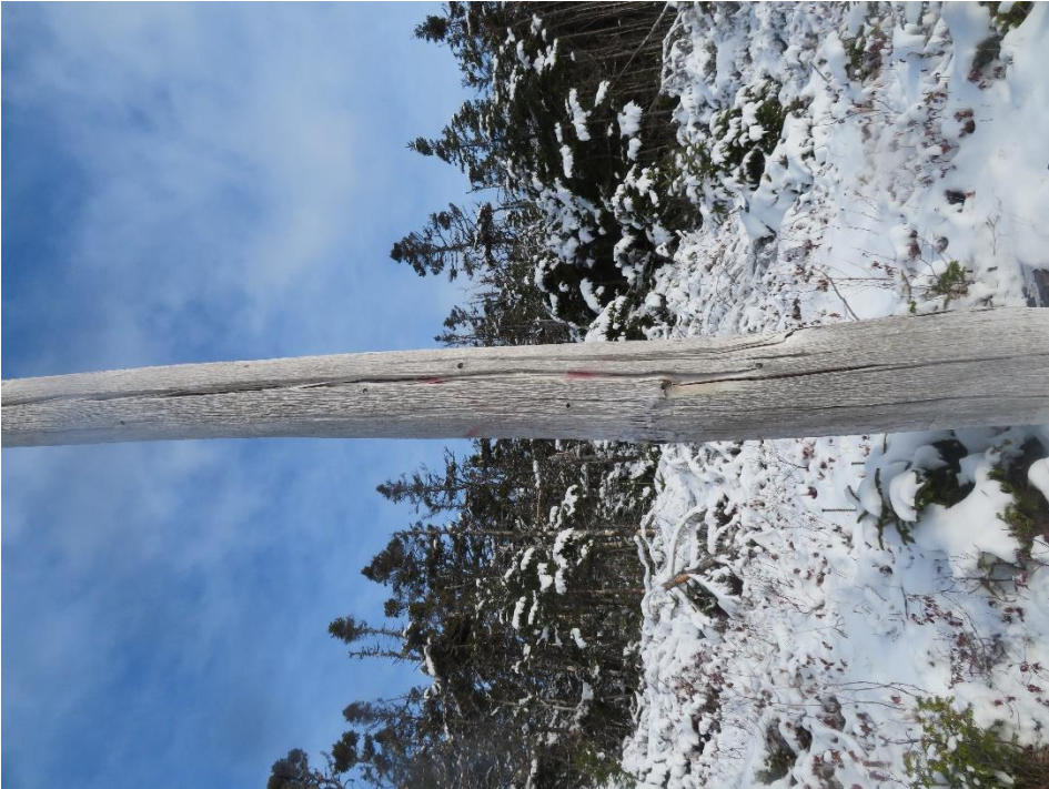
Figure A-9: Deteriorated Pole with Horizontal Split
